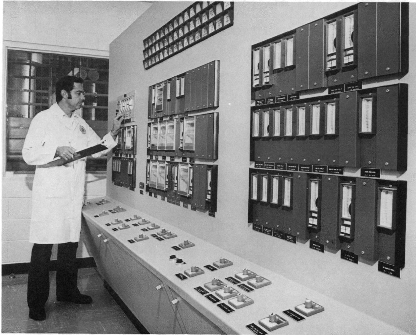
Fig. 2-3. Control panels for circulator test facility
