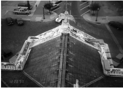
Key: 6-1-3 Roof and dome damage.tif
