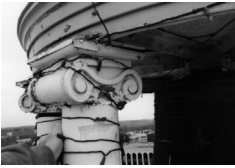
Key: 6-1-2.5ii Damage by wonderland.tif
