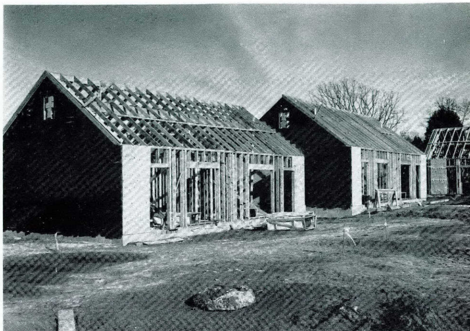
First phase of a $750,000 medical resident center is now under construction. The project consists of seven buildings that will house 20 singles and three families and is expected to be completed this summer.
