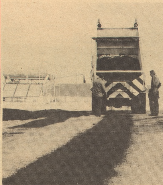
Photo shows how a thin swath of material can be applied using "the box."
