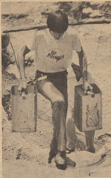
Water to mix the cement for the losa of the latrine is carried to the site by an AMIGOS volunteer.
