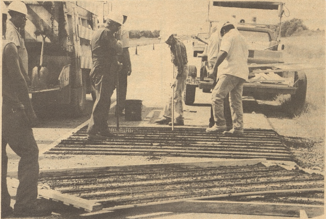
Beaumont District crews apply asphaltic concrete material in Pattern "A" rumble strip on Interstate 10 shoulder. (Photo by Janet Manley)
