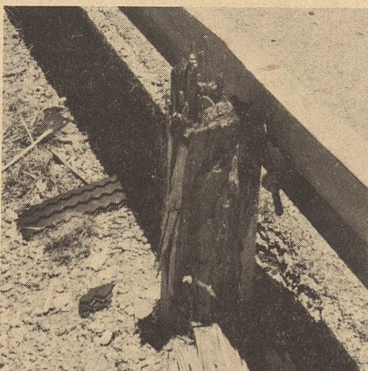
Shattered post protruding slightly above the rail may help deceleration.
