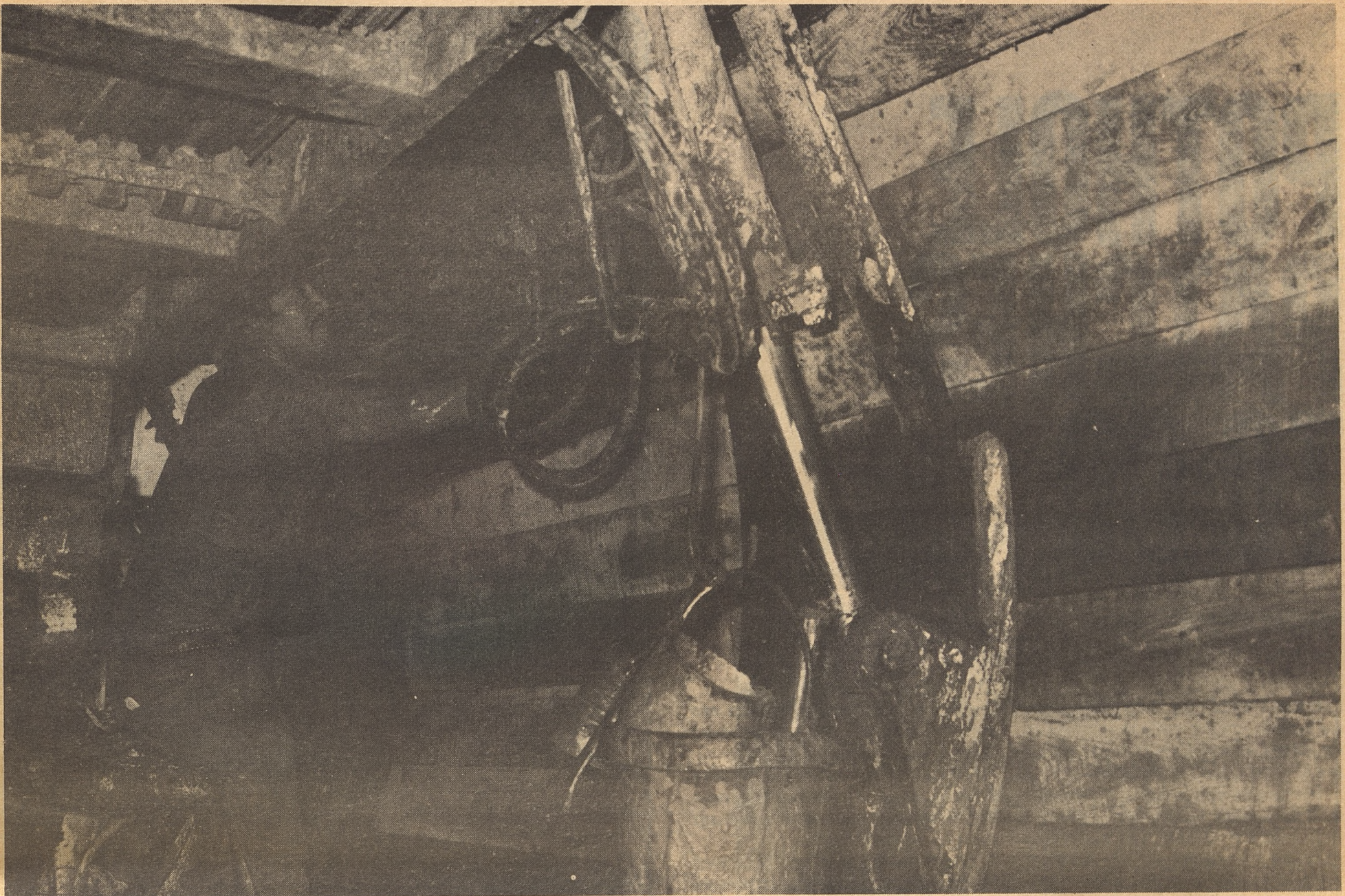
A tunnel can be dug only a little at a time. Using the lagging as a brace, the mole is driven forward five feet by hydraulic pistons. Then the crew sets the rings and puts the new oak lagging in place. The $400,000 mole is then braced against the new lagging and cuts forward again.
