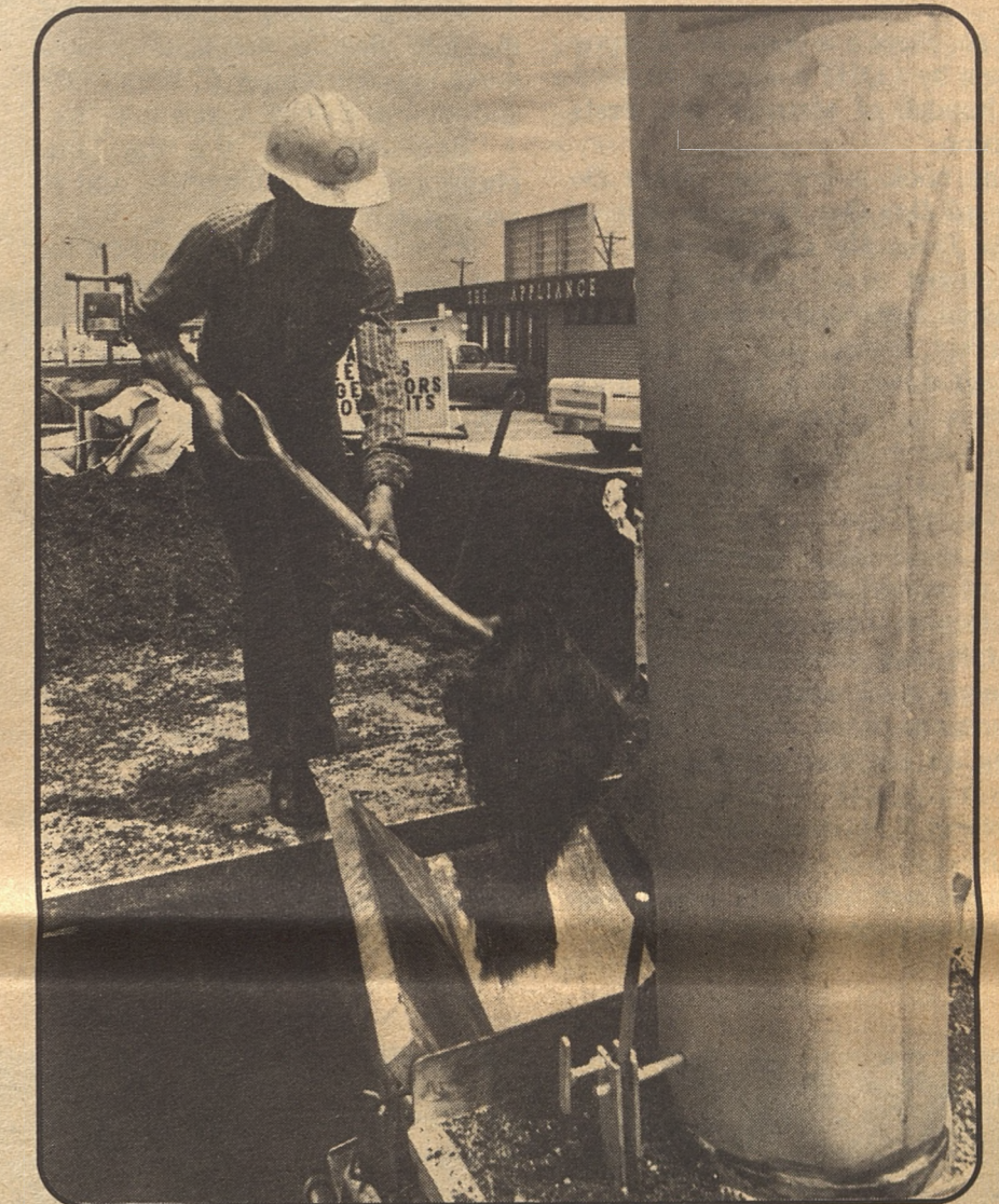
With the Porta-Patcher hitched to the dump truck, old salvage asphalt pavement material can be shoveled directly into the hopper.
