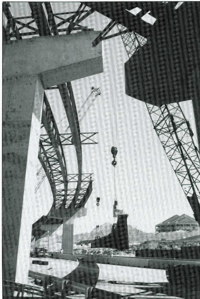
New Interstate 10 interchange is under construction on the west side of El Paso.
