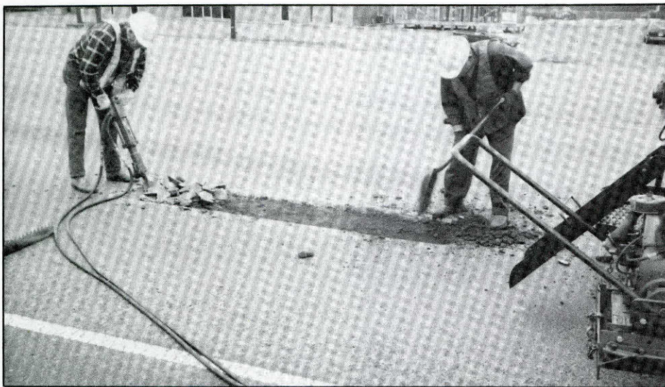
Maintenance operations like this pothole-patching project are undertaken to maintain the integrity of the highway system.
