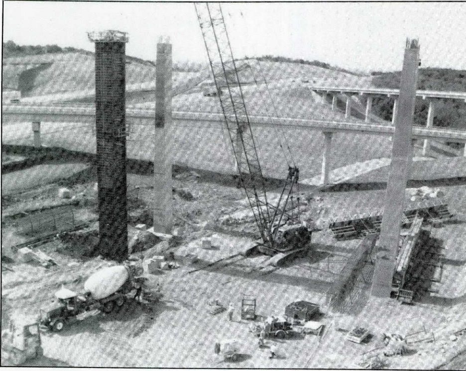
When completed in December, this overpass connecting Spur 408 and Clark Road will provide a north-south traffic corridor for motorists traveling in southwestern Dallas County.
