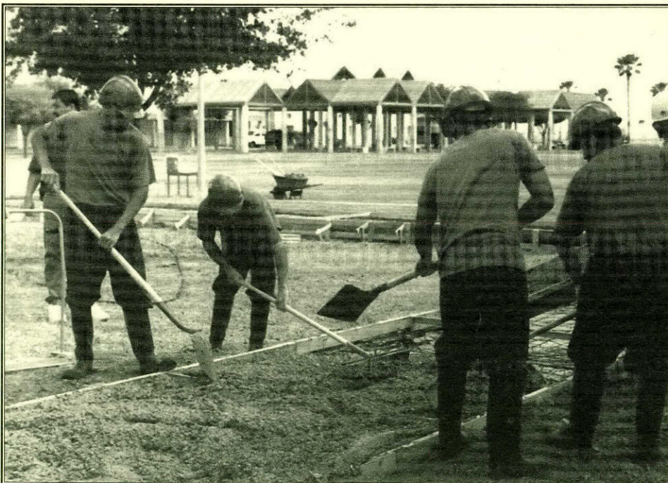
Under the direction of Instructor Robert Flores, Evins Regional Juvenile Center students spread concrete on a sidewalk as part of a building trades construction project. The finished sidewalk connected an area from the infirmary to the cafeteria. The project is one of several scheduled this year. Most notably, the students will be building frame homes for low-income families in the area.
