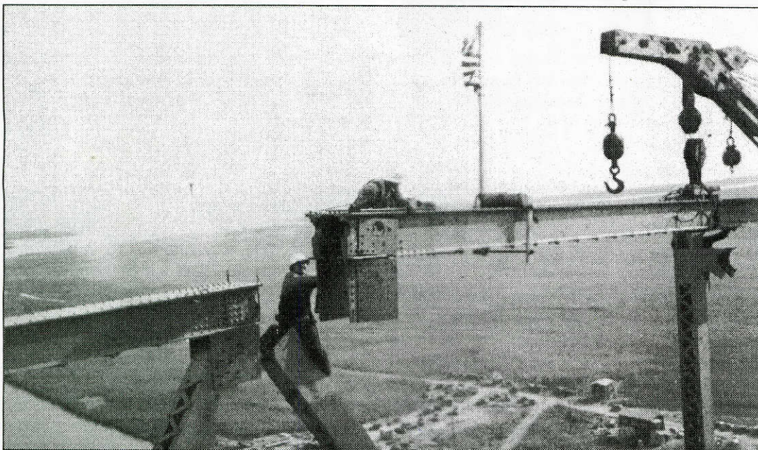
Workers labor to join two cantilevers during construction of the Rainbow Bridge between Port Arthur and Bridge City. The bridge was completed in 1937.
