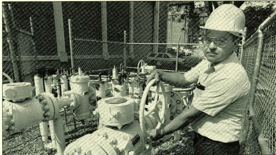
Louis Zschiesche of the Utilities Division adjusts a valve on the university's natural gas pipeline, which recently won a national award.
