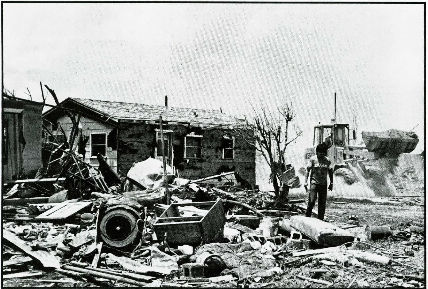
State and local agencies assisted in clearing debris from the community of Saragosa in Reeves County following a May tornado. The Texas Department of Highways and Public Transportation spend about 4,450 personnel-hours at a cost of $75,000. The crews removed 15,845 cubic yards of debris so that the site could be cleared for rebuilding homes. Story, page 2.
