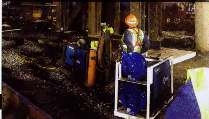
TxDOT crews in the Atlanta District worked through the night constructing a shoring tower for a U.S. 59 overpass in Jefferson after two trains collided and knocked down a supporting column. No one was injured in the collision.
