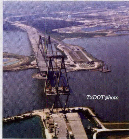
Aerial view during construction of the Hartman Bridge over the Houston Ship Channel.
