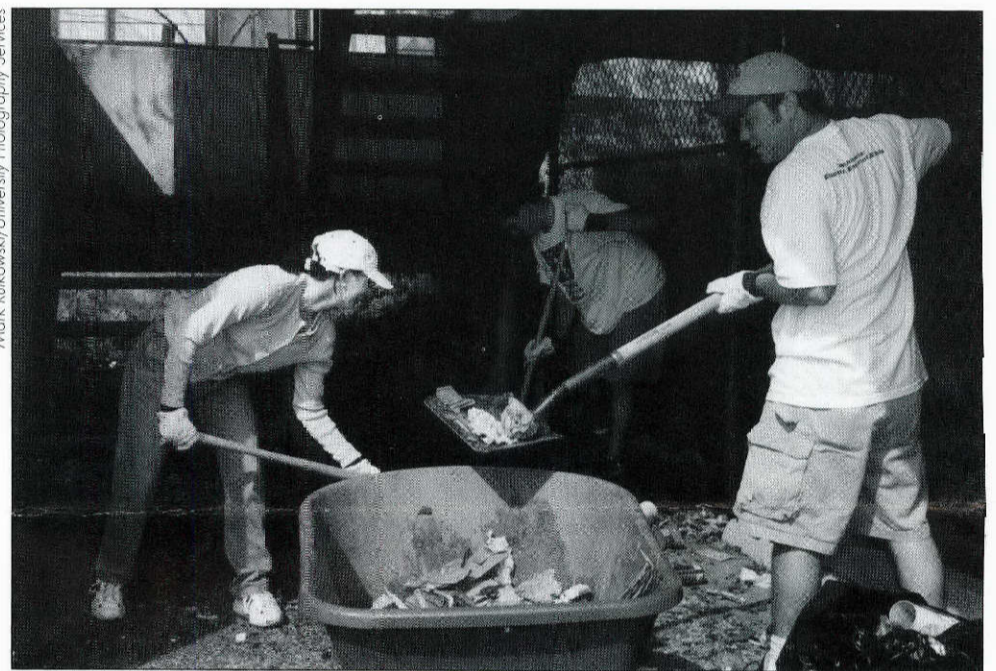
Wendy Block, Kerry Miller, and Drew Murray (left to right) were among the Community Service Day volunteers who helped the city's Neighborhood Housing and Community Development Office clean an abandoned building in East Austin.
