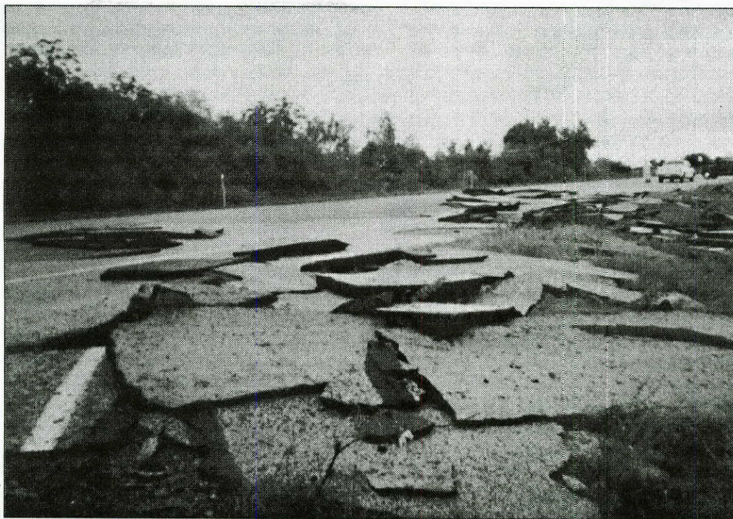
U.S. 77A over Mustang Creek in Lavaca County shows the results of flood damage sustained in April.
