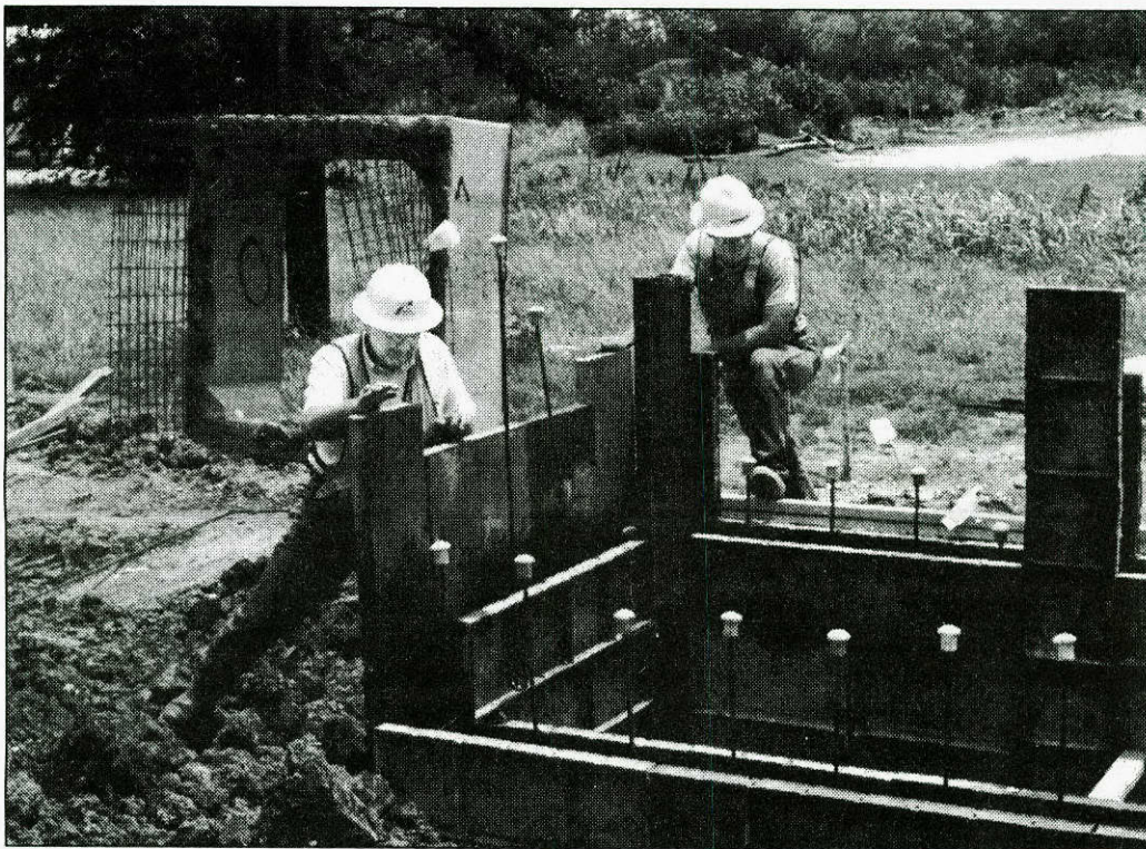
Tyler District construction inspector Jerry Williams, left, and contractor Gregg Kramer inspect a storm sewer inlet. Williams says he believes that his job, like life, should be enjoyed. "If you can't enjoy life, then it ain't worth living."
