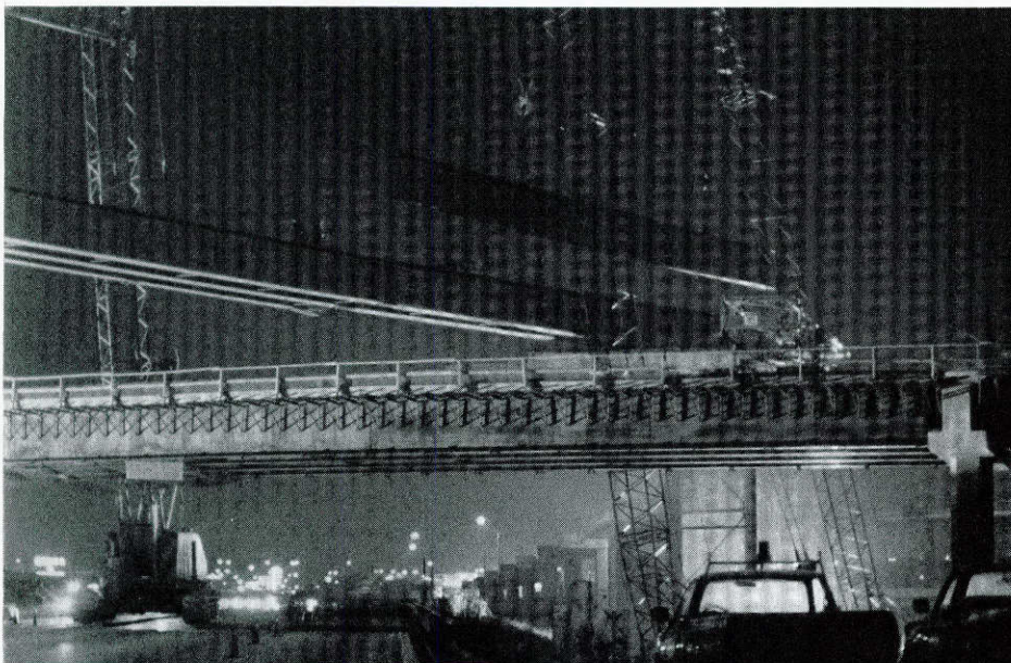
Outlined by the nighttime glow from city lights and traffic, bridge beams are moved into place on the interchange project at US 183 and Loop 1 in Austin. The $38 million, four-level interchange will be completed in 1990.
