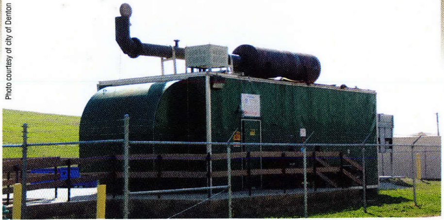
Methane collected at the Denton landfill is transferred to an onsite 1.6-megawatt electric power generator system, which sends enough electricity back to the municipal utility company to power about 1,600 homes daily.
