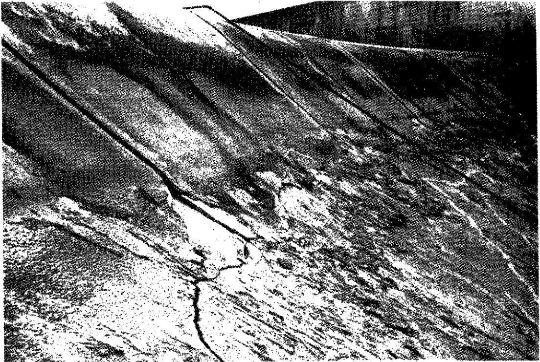
Downstream View of Spillway Showing Cracks at Base of Hollow Buttress Weir. (Note Book and Cigarette Package.)
