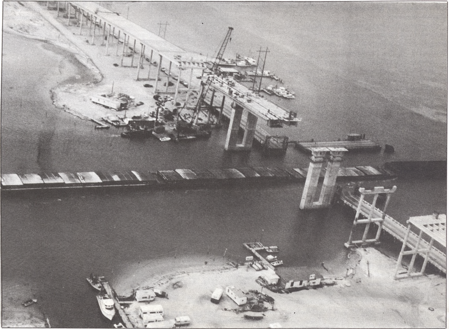
Barge traffic in the Gulf Intracoastal Waterway continued without disruption during construction of the JFK Causeway, which opened in 1973. The causeway recently won recognition as the first precast segmental bridge in the United States. (Photo by Jim Allen, Materials and Tests Division)
