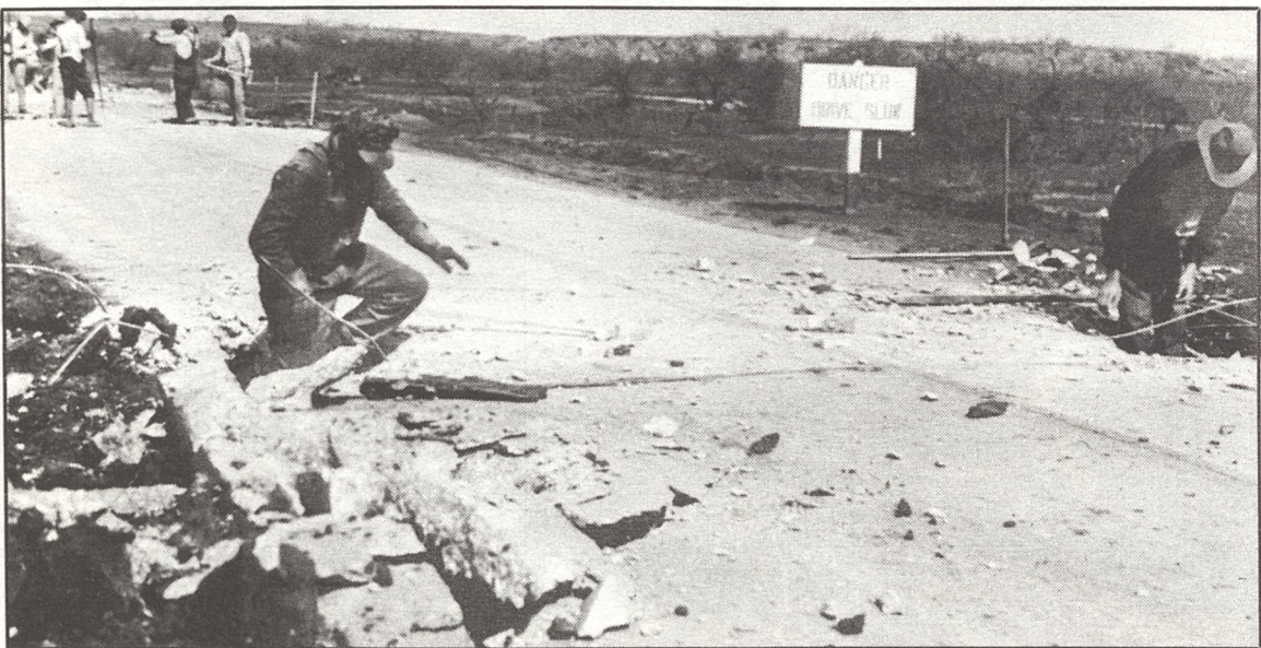
"Danger — Drive Slow" said the sign along Texas 79 in Archer County in 1931. No kidding. Maintenance forces had to use a half stick of dynamite at each slab corner to break up the damaged concrete. The rest was removed with drills and sledge hammers.
