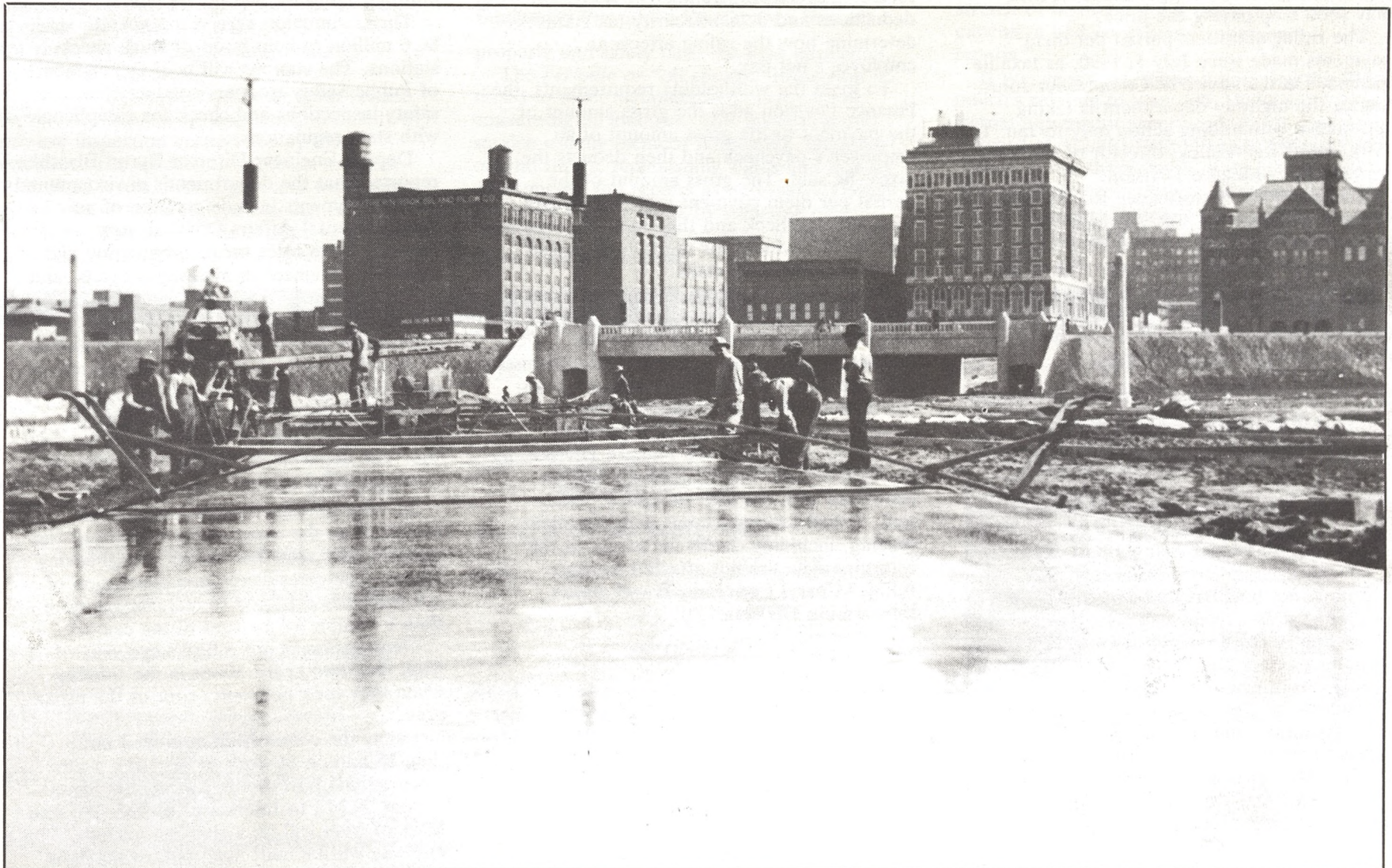
In 1936, Commerce Street in Dallas was being laid in concrete just west of the Southern Pacific Railroad and the "triple underpass." The fancy building on the right is the old courthouse; the tallest building visible on the left became the infamous Texas Schoolbook Depository.
