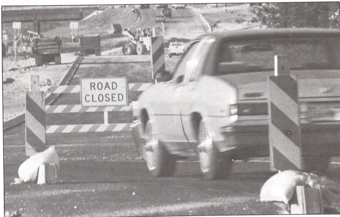
Construction scenes like this may become scarce if highway funding is not renewed by Congress in 1991. Authorization for three major components of the national highway program expires Sept. 30, 1991, and transportation advocates across the country are working for a consensus policy. (Photo by Jack Lewis, Travel and Information Division)
