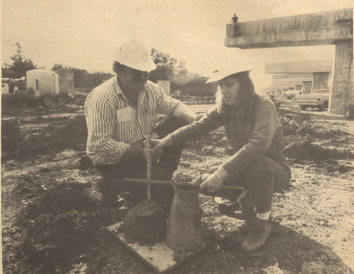
Lisa Grose of the Highway Design Division works with Mike Palmer of the South Travis County residency on a "slump test," which determines the amount of moisture in concrete. (Photo by Kevin Stillman)
