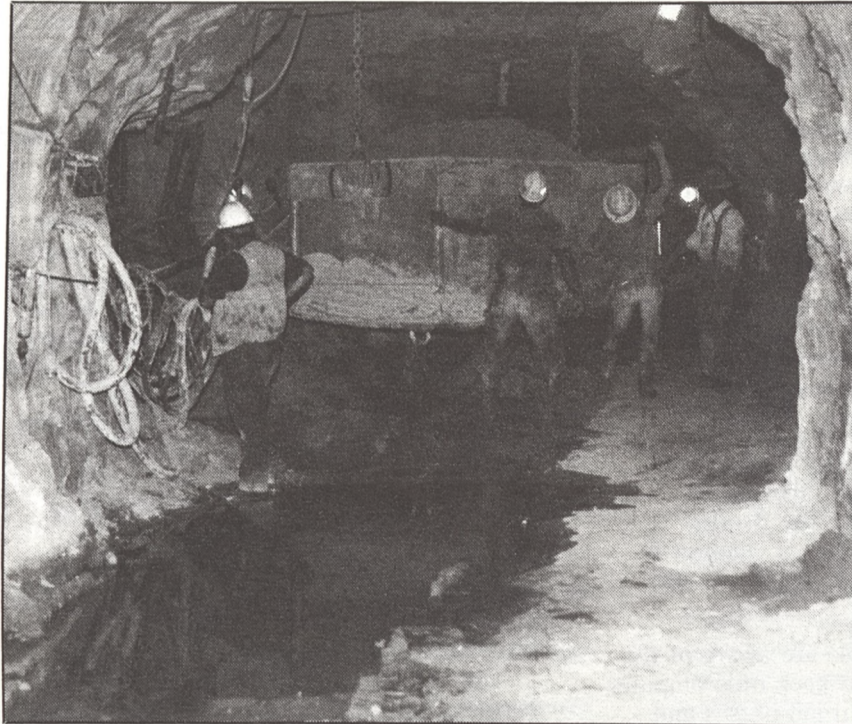
Work goes on continually to dispose of the tons of chalk produced by the machine boring Dallas' largest drainage tunnel under North Central Expressway. (Photo by Juan Carlos Reynoso, Dallas District)
