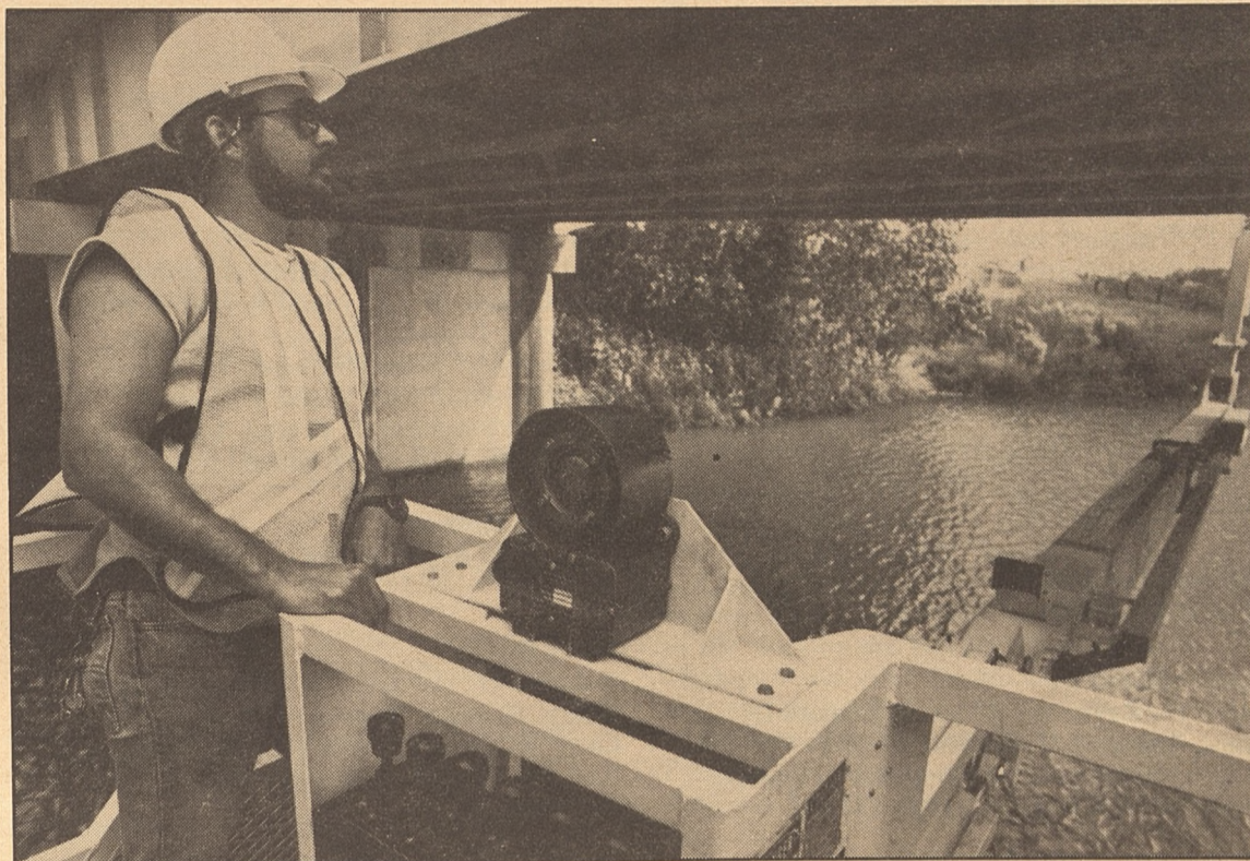
Bruce Sims of D-4 demonstrates the full reach of the UB60 under the LaSalle bridge over Lake Brazos in Waco. (Photo by Kevin Stillman, Travel and Information Division)
