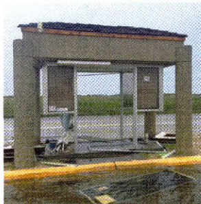
Mustang Island State Park sustained significant damage to roads and buildings. →
