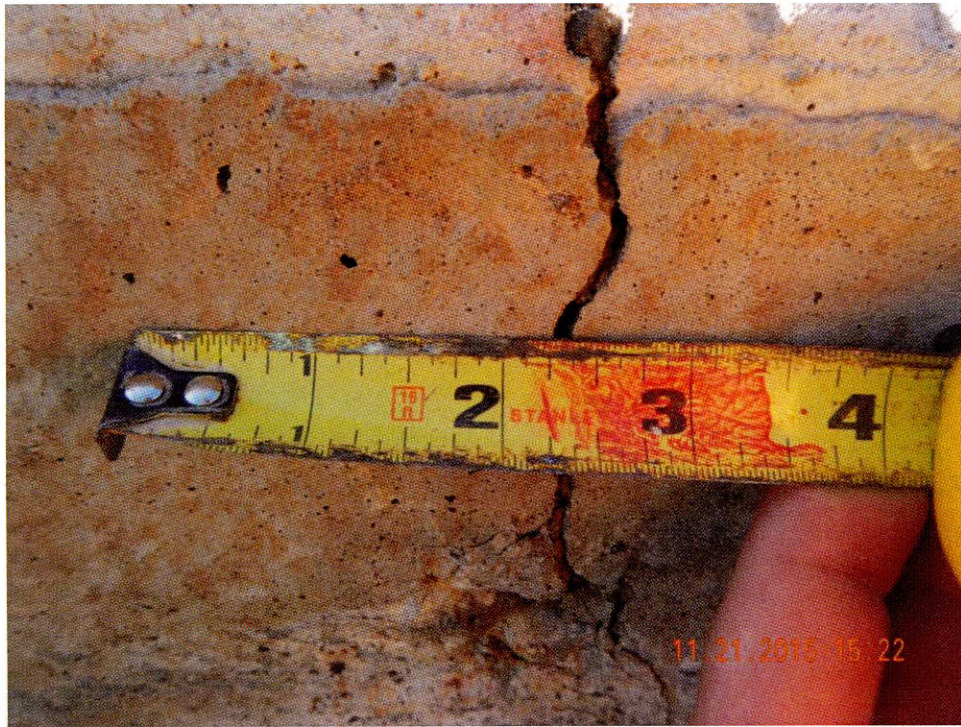
Figure 4.24 Crack width at Joint on FM 2253
