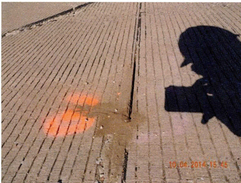
Figure 2.5 High level of stone intrusion
