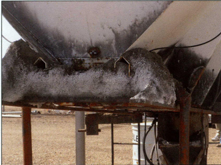
FIG 36. The main corrosion concern to infrastructure is the corrosion of ferrous metals
