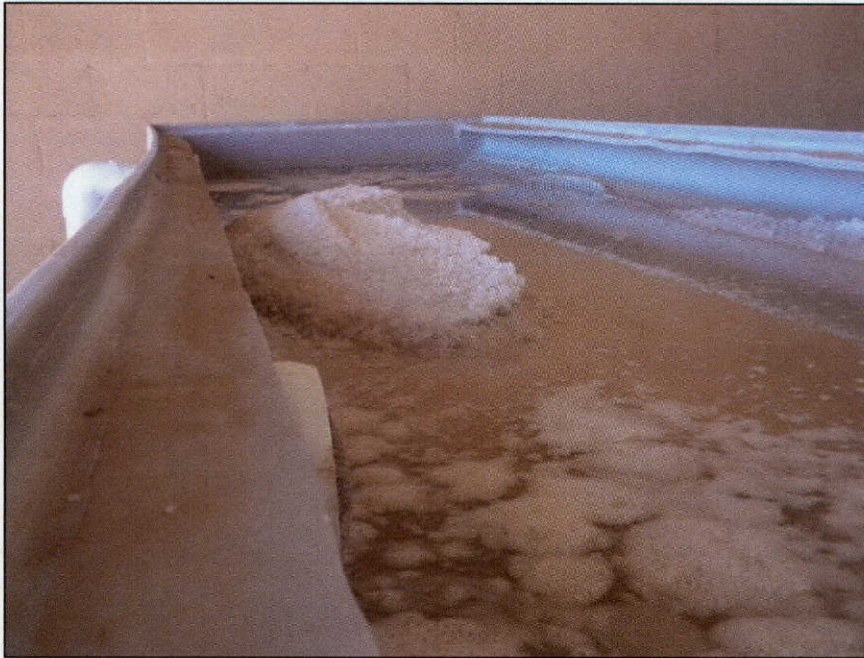
FIG 17. The TxDOT Childress District invested in a salt brine manufacturing tank system to make their own salt brine
