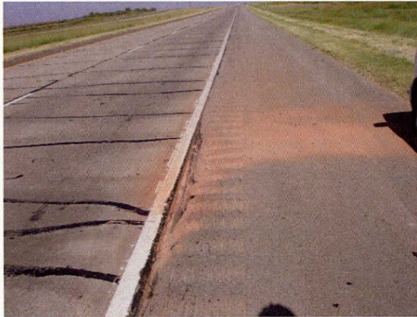
Figure 4.1 Severe Pumping at The Edge of Pavement with Asphalt Stabilized Base
