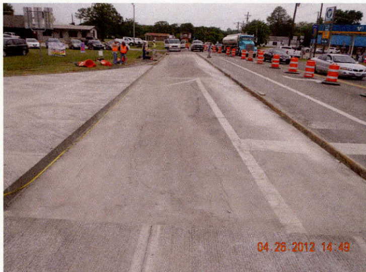
Figure 3.2 Distress on Existing Asphalt Pavement.
