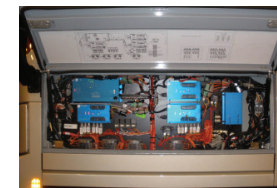
Multiplexing Electrical System
