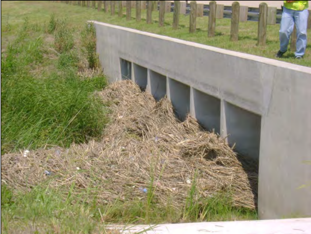
Figure 4. Illustrating the debris collecting at the downstream end of the culvert at Airfield Drive.
