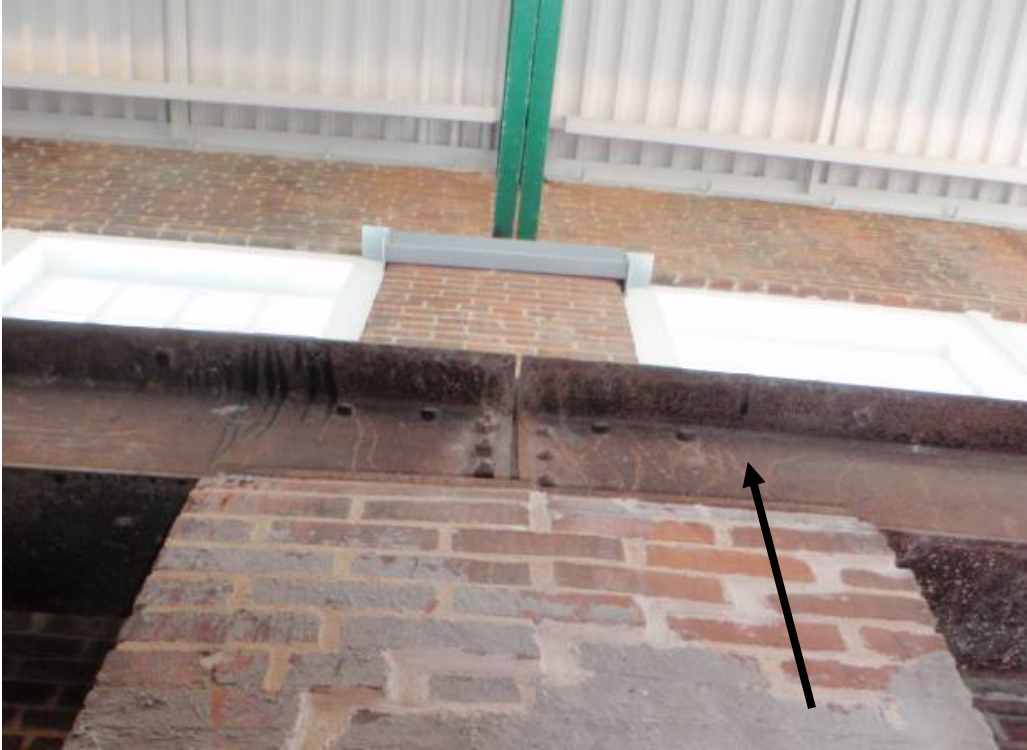
Figure 21: Crane Rail Support Beam
