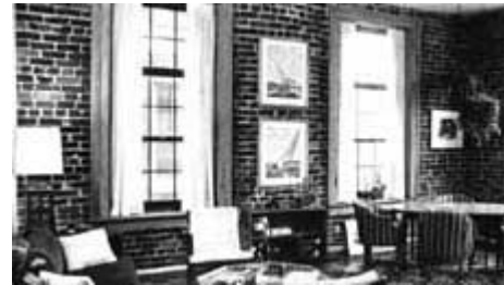
Plaster has been removed from perimeter walls, leaving brick exposed. The plaster should have been retained and repaired, as necessary. Photo: NPS files.
