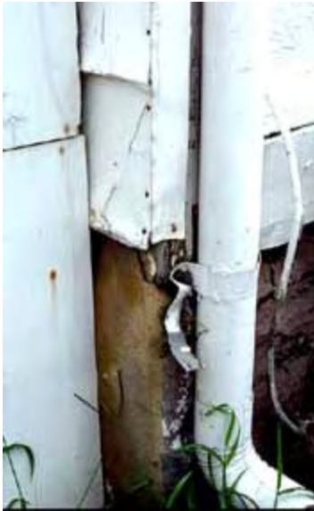
A clogged or broken downspout causes the water to pour directly into the ground. NPS files. Photo: NPS files.
