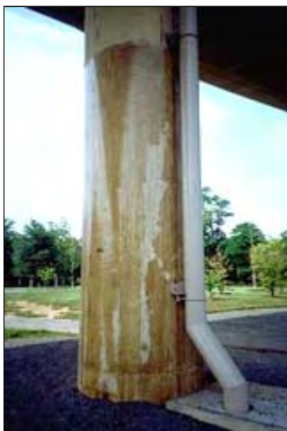
This formerly clear barrier coating is very shiny and has discolored as it has aged. Photo: NPS files.
