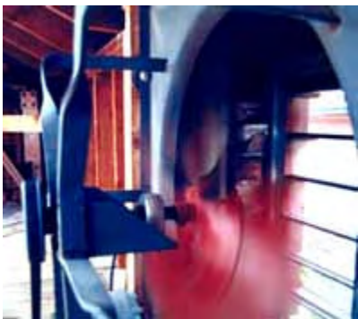
Installing ventilating fans can improve damp conditions or reduce cooling loads. Photo: NPS files.
