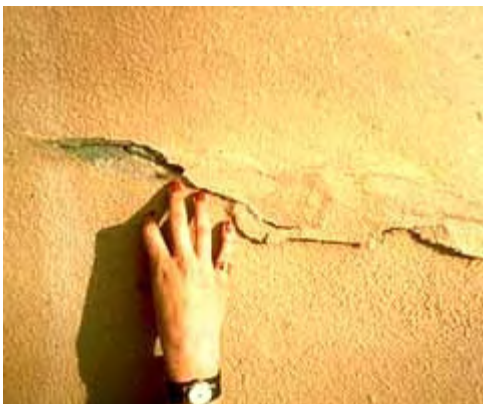
Applying a waterproof coating to an above-ground masonry wall can trap moisture underneath, causing further damage to the historic material. Photo: NPS files.
