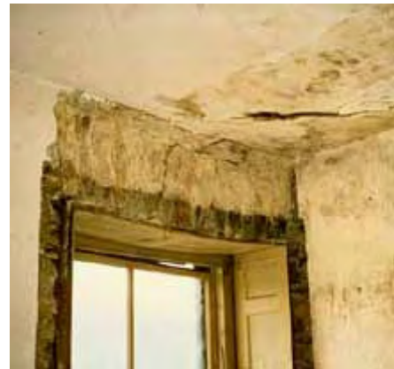
Damp interior plaster around windows generally indicates moisture has entered from the outside. Photo: NPS files.
