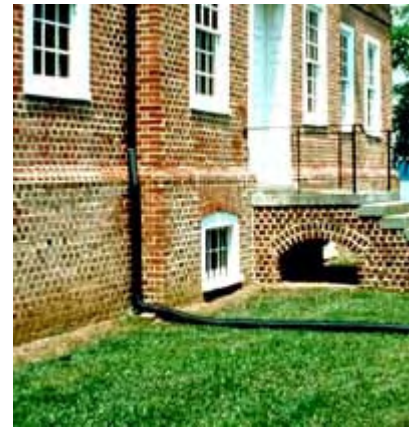
The owner used long black extender pipes to test a theory that it was faulty roof drainage causing the problem. Photo: NPS files.
