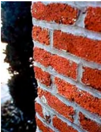
Abrasive cleaning can cause permanent damage to historic fabric, such as this brick wall. Photo: NPS files.
