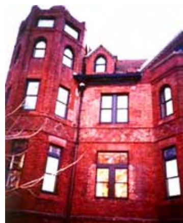
Unskilled repointing has negatively impacted the character of this late-19th century building. Photo: NPS files.
