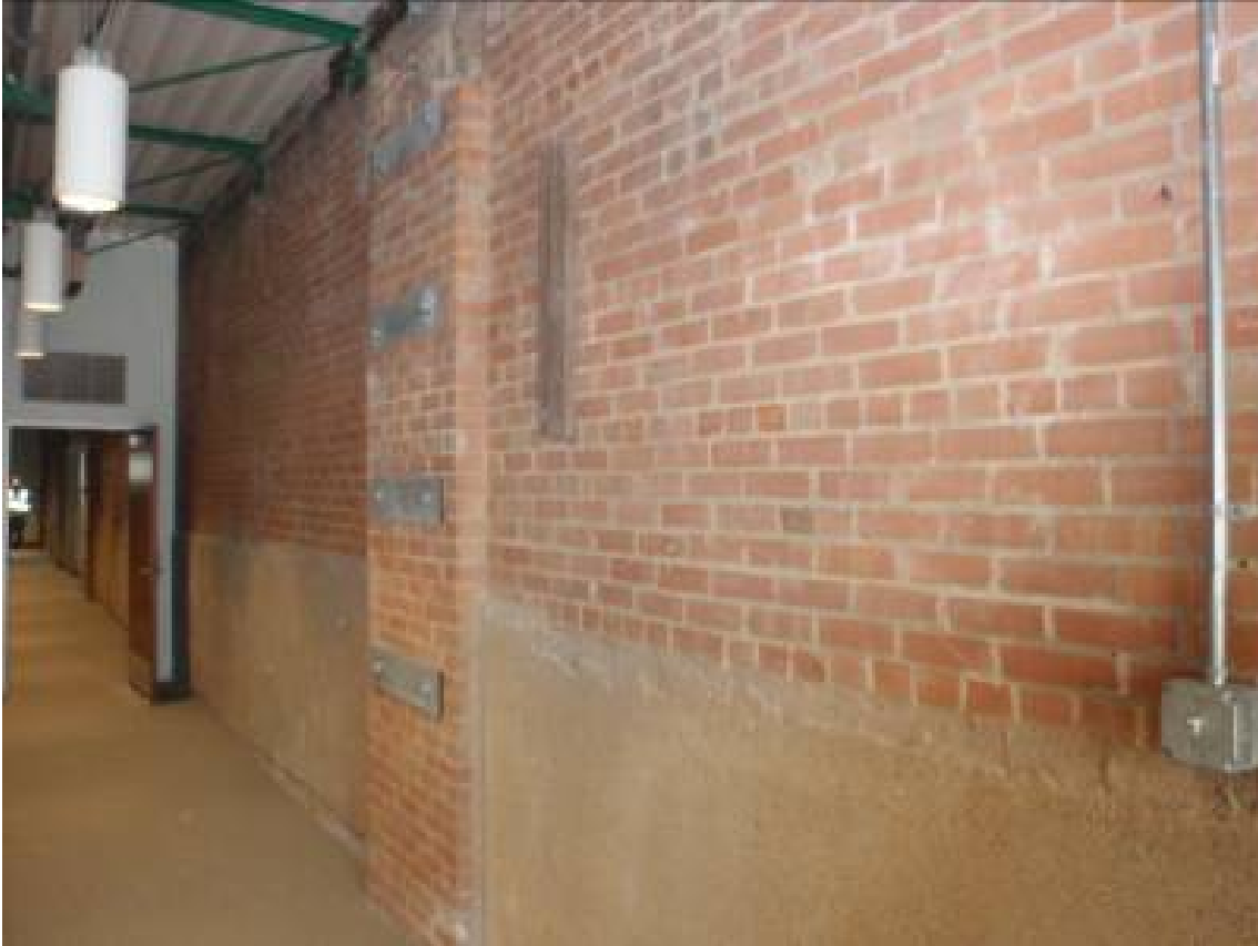
Figure 27: Interior Brick Wall on second floor runs north to south in the building
