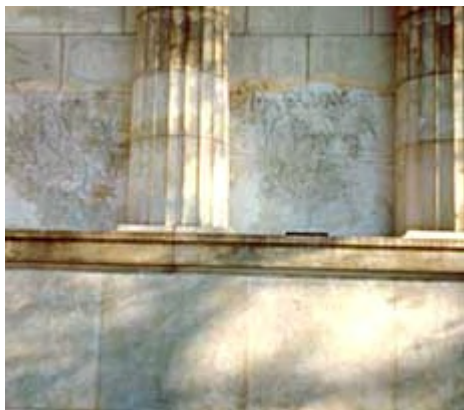
Damaging graffiti removal methods have scarred the marble. Photo: NPS files.
