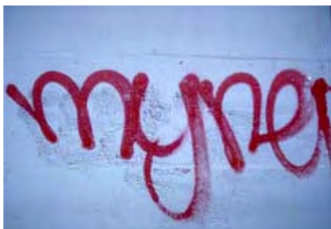
Inappropriate abrasive blasting to remove the graffiti has permanently etched the graffiti into the stone. Photo: NPS files.
