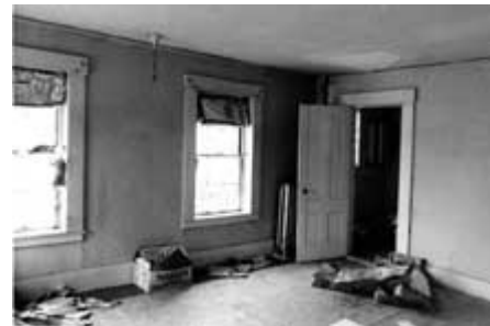
The interior of this 19th worker's house has not been properly maintained, but it may be as important historically as a richly ornamented interior. Its wide baseboards, flat window trim, and four-panel door should be carefully preserved in a rehabilitation project. Photo: NPS files.
