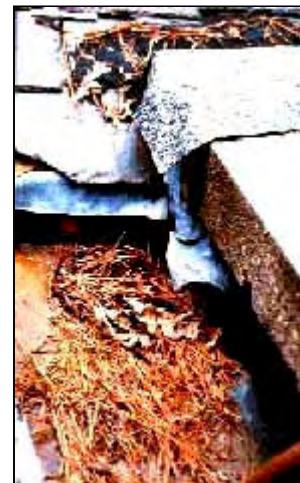
Debris will impede the normal flow of water from the roof's gutter and downspout system to the ground and result in moisture problems. Photo: NPS files.
