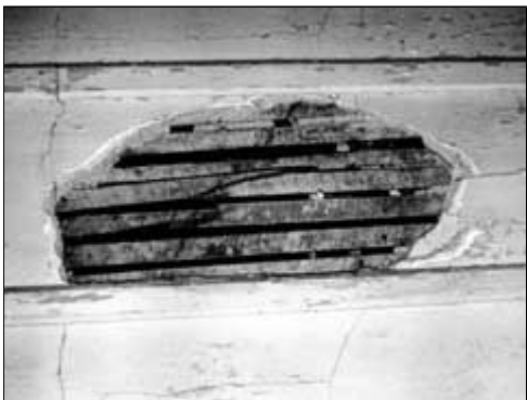
This beaded ceiling in one of the bedrooms of the 1847 Lockwood House, Harpers Ferry, West Virginia, is missing portions of plaster due to broken keys. Photo: NPS files.
