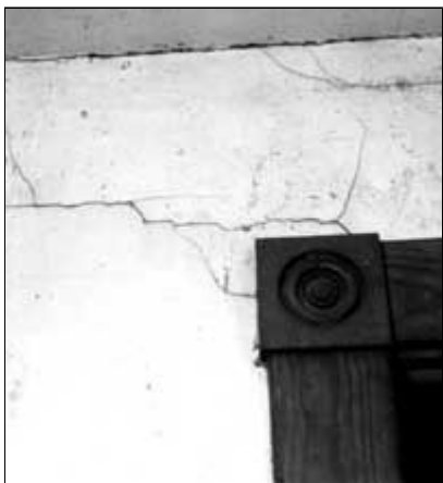
Stress cracks in plaster over a kitchen door frame can be repaired using fiberglass mesh tape and joint compound. Photo: NPS files.
