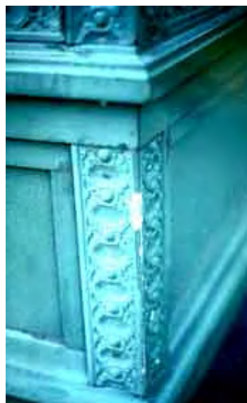
Substitute materials need to be located with care to avoid damage. The fiberglass column base has chipped, whereas the historic cast iron would have remained sound. Photo: NPS files.
