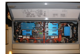
Multiplexing Electrical System
