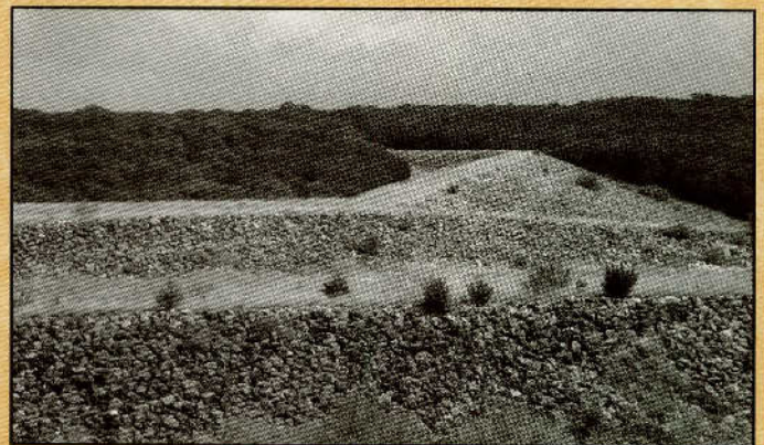
The Krause's Dam is one of three recharge dams on the western arm of Dry Comal Creek to help prevent flooding.
