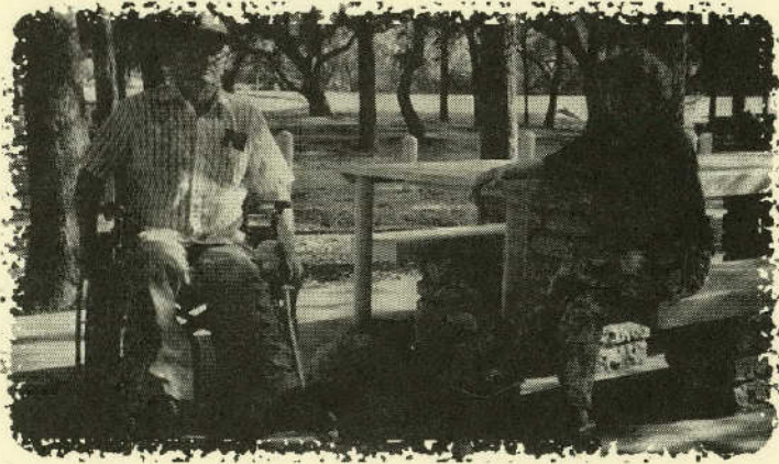
Picnic table extension installed to make it possible for people in wheelchairs to sit comfortably. Photo courtesy of Katy Kalk, TxDOT
