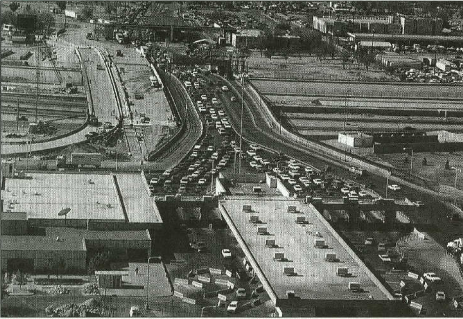
Under construction—the Cordova International Bridge of the Americas joining El Paso, Texas and Ciudad Juarez, Mexico
