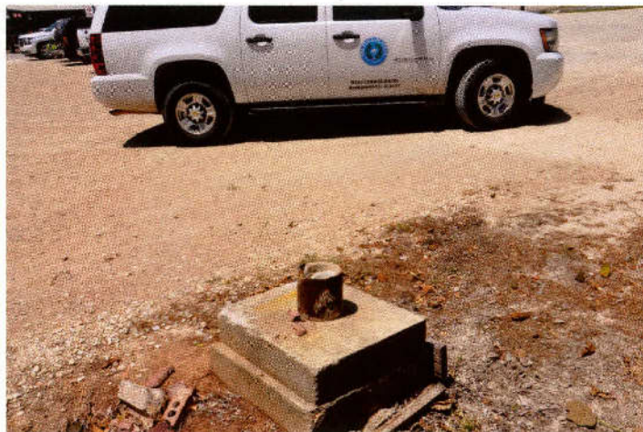
Abandoned, deteriorated, and unplugged water well in an open parking lot near Salado, June 2018.
