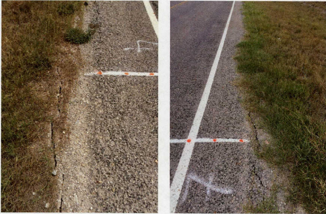
Figure 4.34 Example pictures of the longitudinal cracks developed at the edges of test sections at FM 2924
