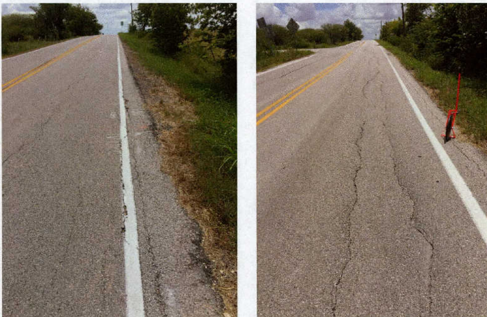
Figure 4.53 Example pictures of longitudinal cracks observed at Turnersville Road test sections in 2017
