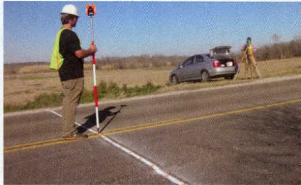
Figure 4.6 Using total station and prism to monitor vertical deformation of the marked transverse sections
