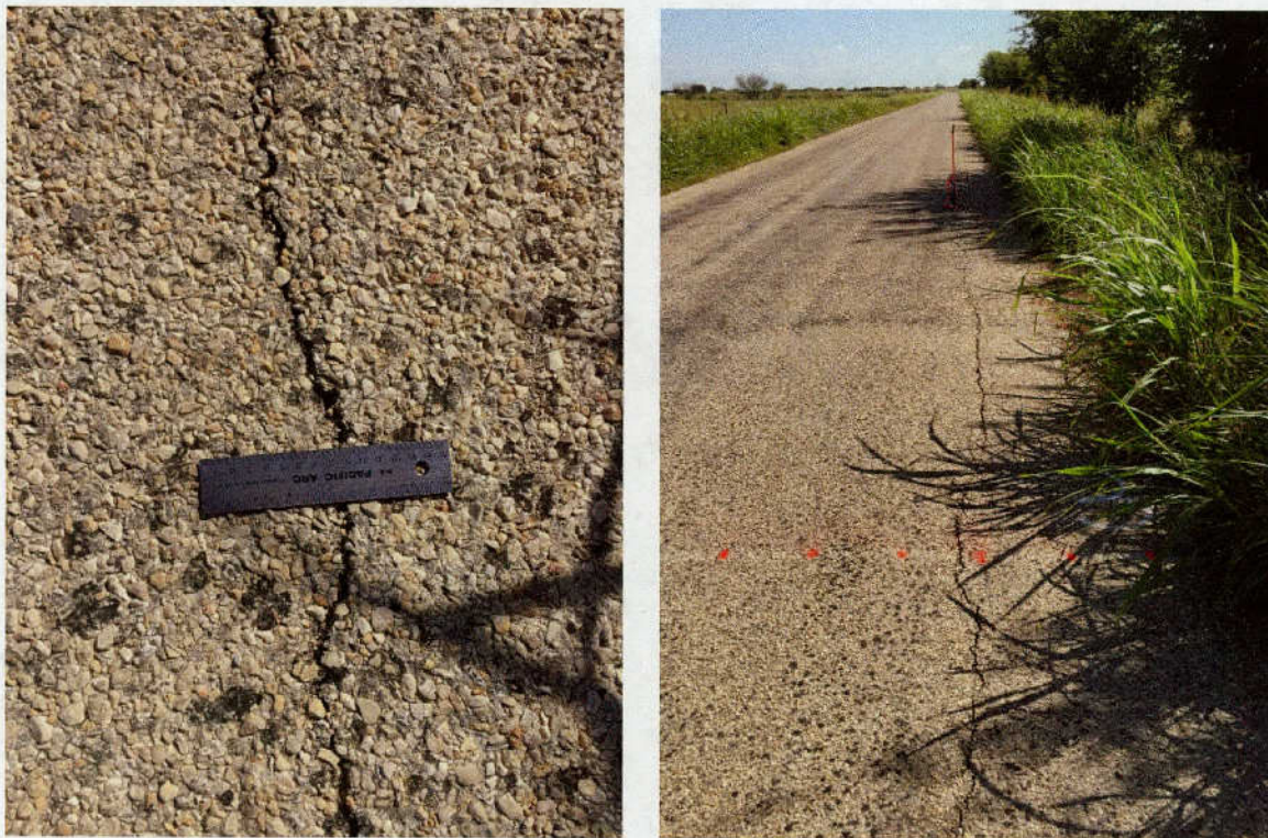
Figure 4.46 Example pictures of longitudinal cracks in control section at Cabeza Rd.
