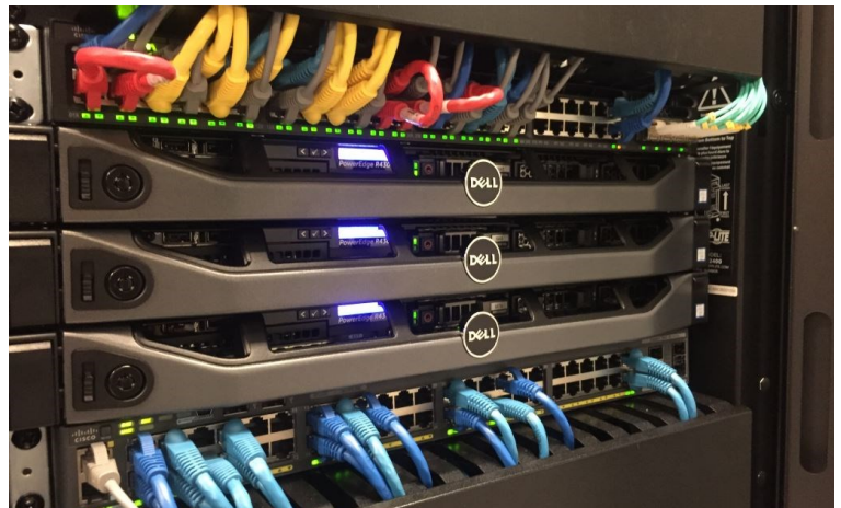
Equipment in CSEC's racks at the Texas DIR facility in Austin.
