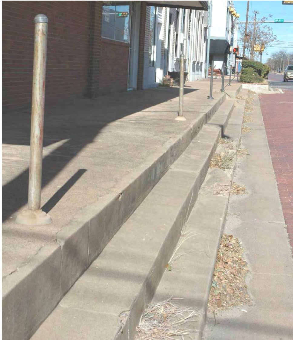
Figure C-33. 100 block of S. Avenue C, Olney. The curbing in this block typifies conditions throughout downtown Olney.
