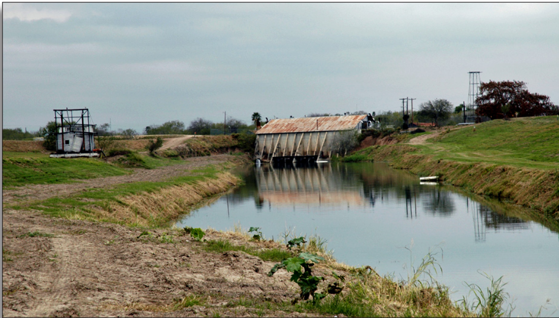
Figure 69: View up inlet looking north towards first lift station, Hidalgo County Irrigation District No. 1.
