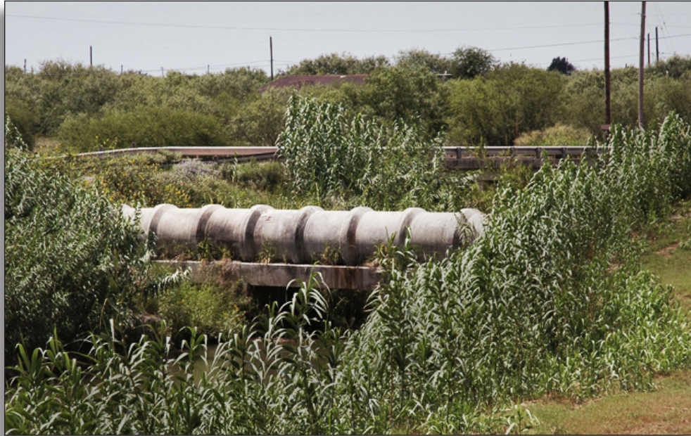
Figure 128: Full-round flume (c.1990) from Lake Edinburg to main canal, Santa Cruz Irrigation District No. 15.
