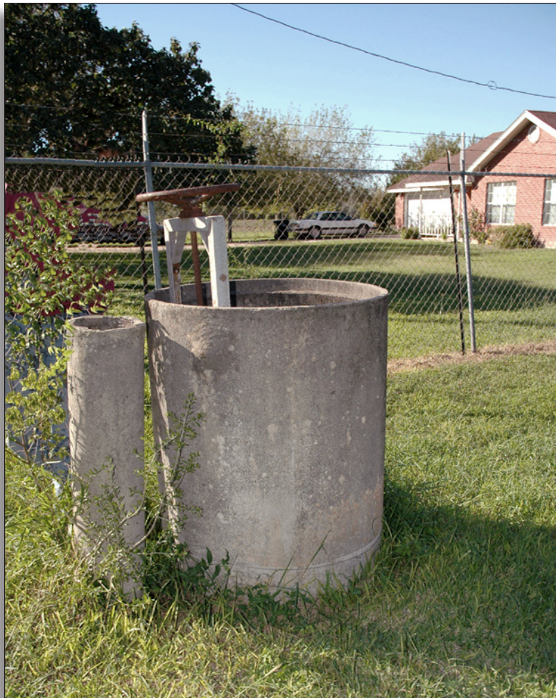
Figure 180: Vent pipe (left) adjacent to diversion stand (right), late 1930s, Cameron County Irrigation District No. 6.
