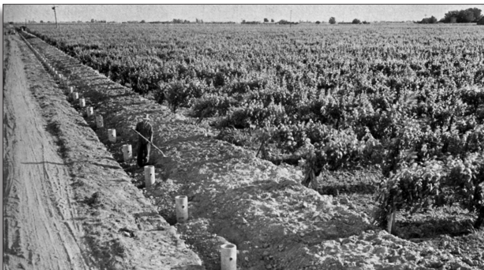
Figure 167: Installation of 8" standpipes to control water flow into furrows (c.1935). Source: Loving, Concrete Pipe for Irrigation and Drainage
