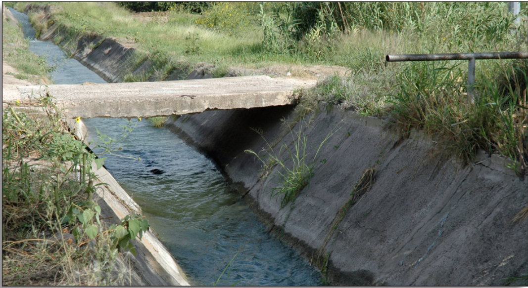
Figure 212: Pedestrian bridge (c.1945) north of Lake Edinburg, Santa Cruz Irrigation District No. 15.
