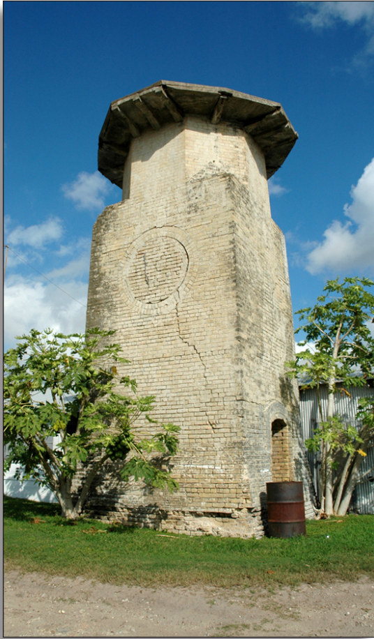
Figure 238: Base of old water tower at first lift station, Cameron County Irrigation District No. 6.
