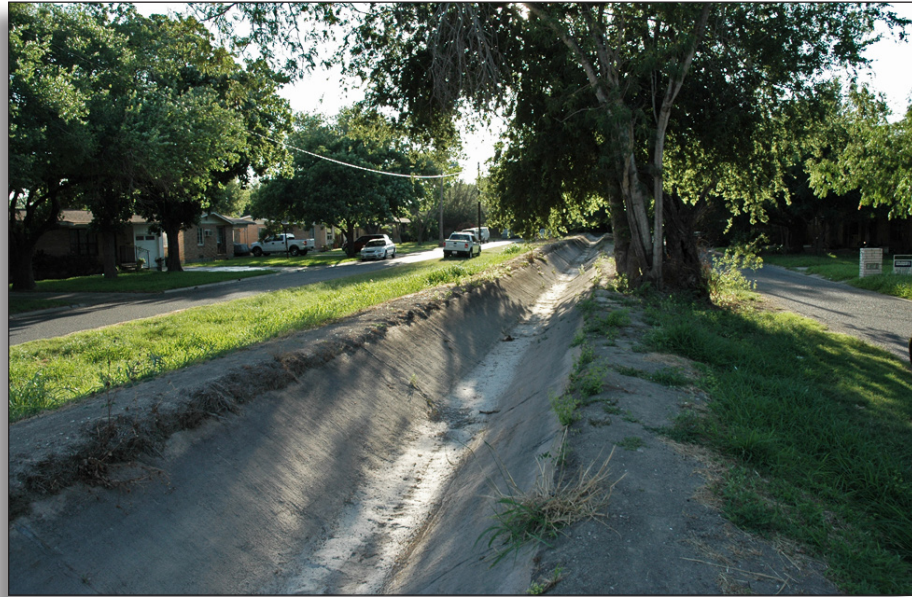
Figure 315: This abandoned concrete lateral in a residential area of McAllen has lost integrity of association, Hidalgo County Irrigation District No. 3.
