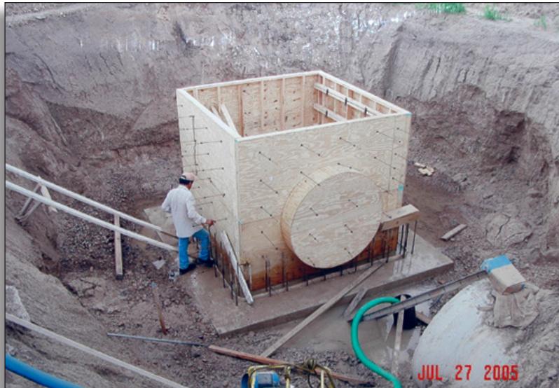
Figure 321: Construction of concrete forms for standpipe, East Main Project (2005). Photo collection, Hidalgo County Irrigation District No. 1
