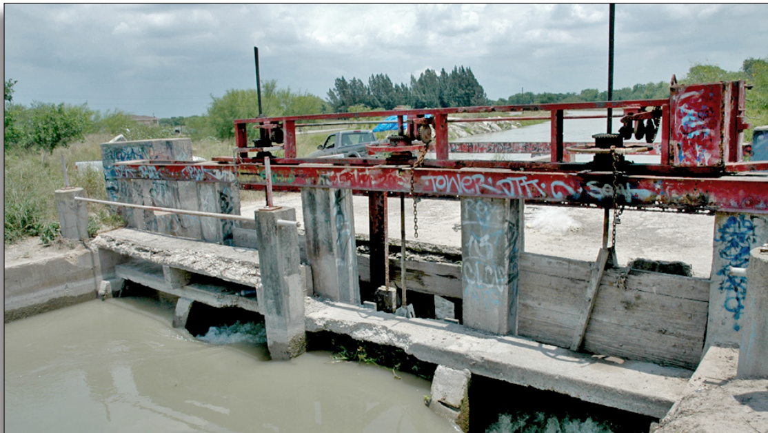
Figure 293: The addition of motorized gates adversely impacts the integrity of materials in this historic-age check gate, Cameron County Irrigation District No. 2.
