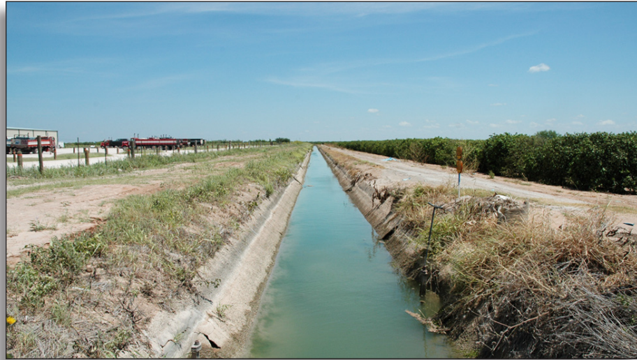
Figure 299: The RL Main Canal has been raised and redesigned to improve water flow, impacting its integrity of workmanship and design, Hidalgo County Irrigation District No. 15.
