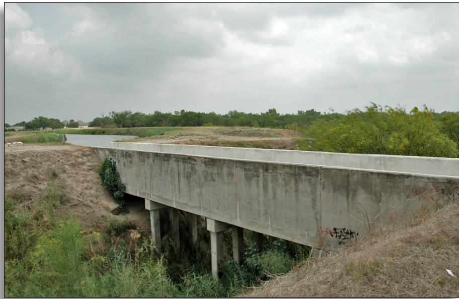
Figure 126: Box flume at floodway (2004), Mission Inlet, United Irrigation District.
