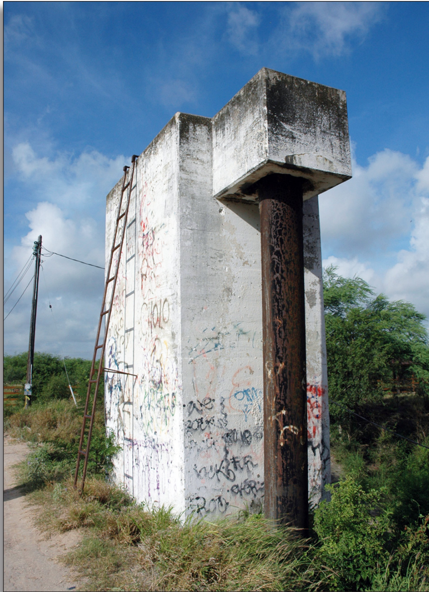
Figure 175: Surge chamber (1948) near Pump No. 3, Santa Cruz Irrigation District No. 15.
