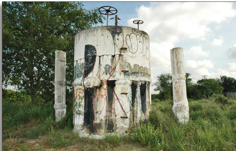
Figure 179: Diversion well (1948), Santa Cruz Irrigation District No. 15.
