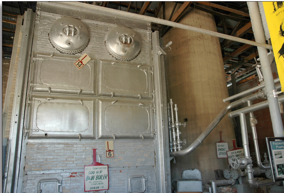
Figure 76: Interior view of boiler room, Old Hidalgo First Lift Pumphouse.
