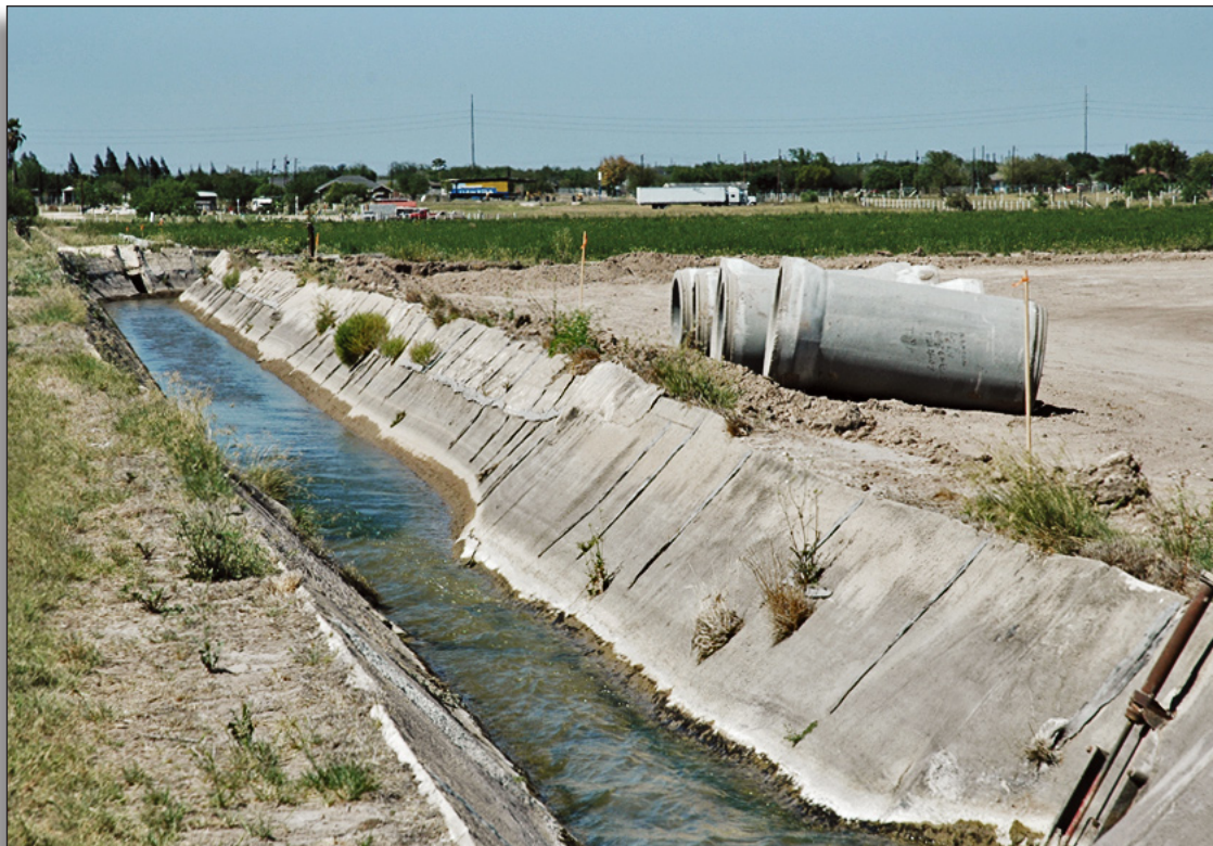
Figure 116: Lateral being placed in underground pipeline along Troser Road, United Irrigation District.
