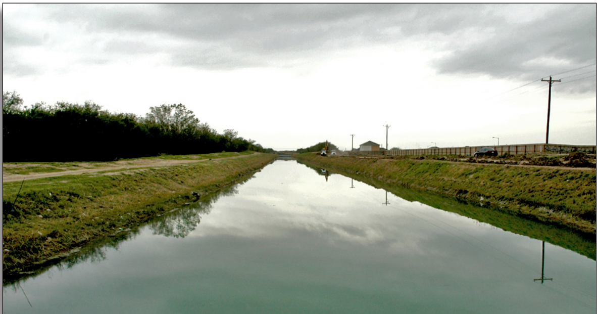
Figure 298: Portions of earthen Edinburg Main Canal maintain integrity of workmanship, but represent only a small segment of the total conveyance system, Hidalgo County Irrigation District No. 1.
