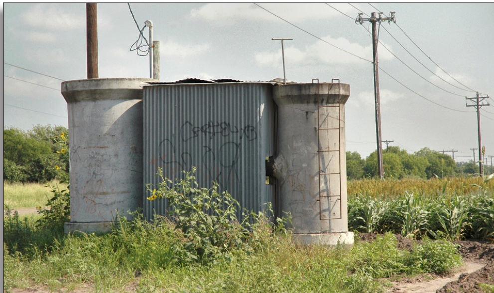
Figure 174: Pump stand adjacent to underground pipeline, FM 803, Old Cameron County Irrigation District No. 13.
