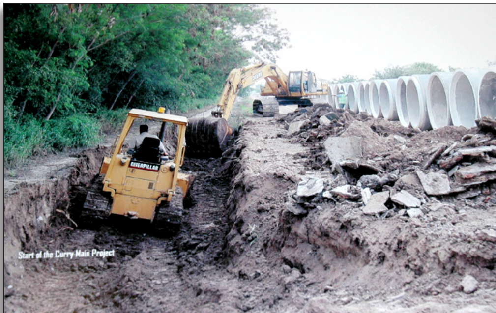
Figure 139: Initial construction of Curry Main Canal project in 2004. Source: Photo collection, Hidalgo County Irrigation District No. 1
