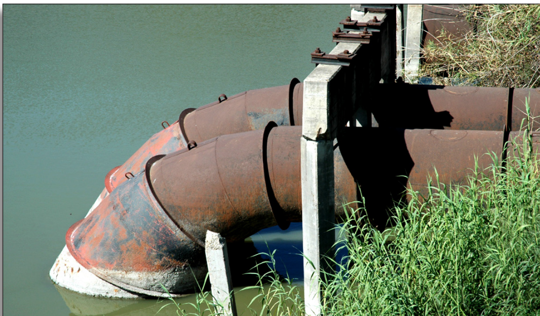
Figure 75: Inlet pipes to first lift pumphouse, Hidalgo County Irrigation District No. 1.
