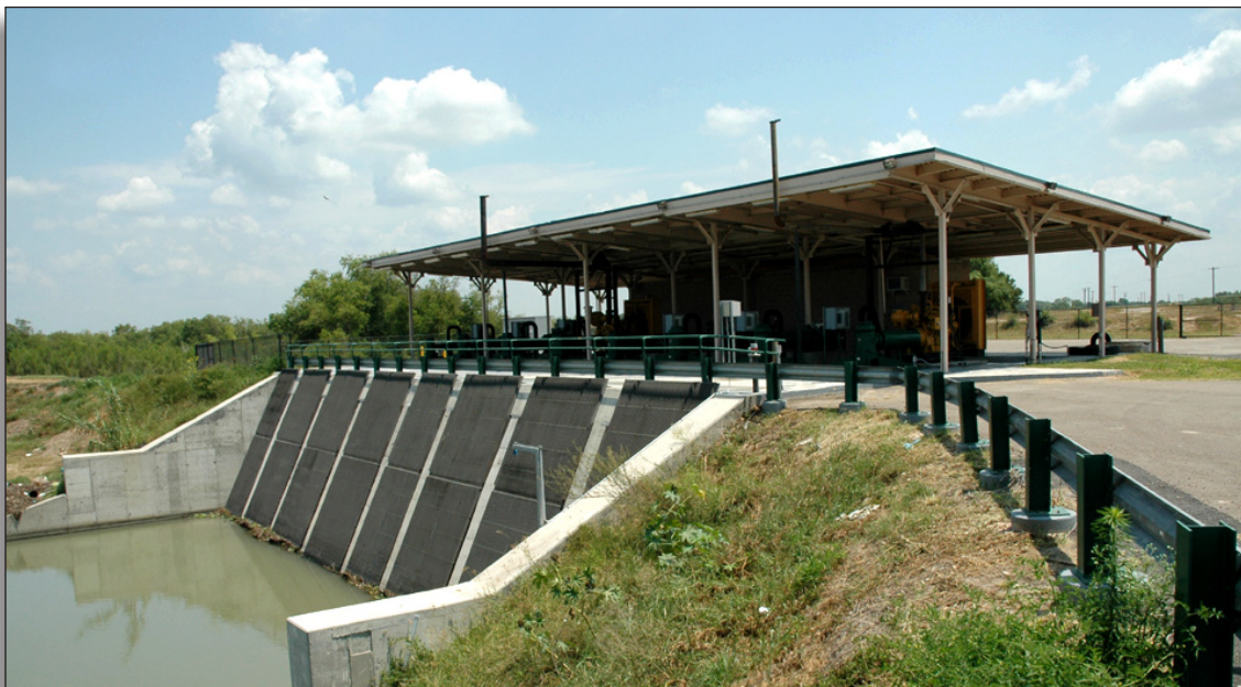
Figure 279: The modern pumping plant (2005) at Los Indios is located north of the old pumping plant and required a realignment of the main canal.
