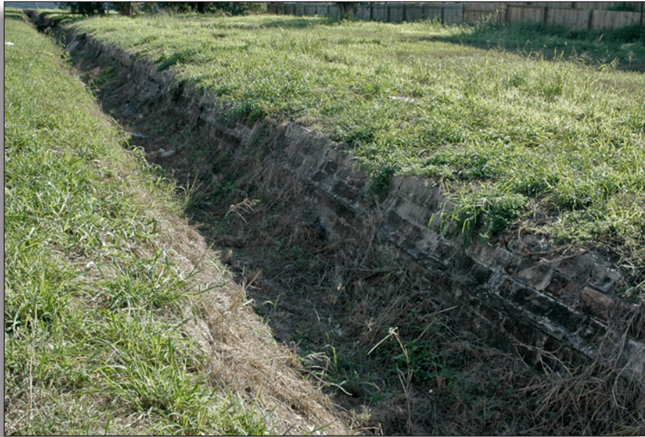
Figure 119: Brick lined Stub-Tandy Lateral (1938), adjacent to Tandy Road, Cameron County Irrigation District No. 6.
