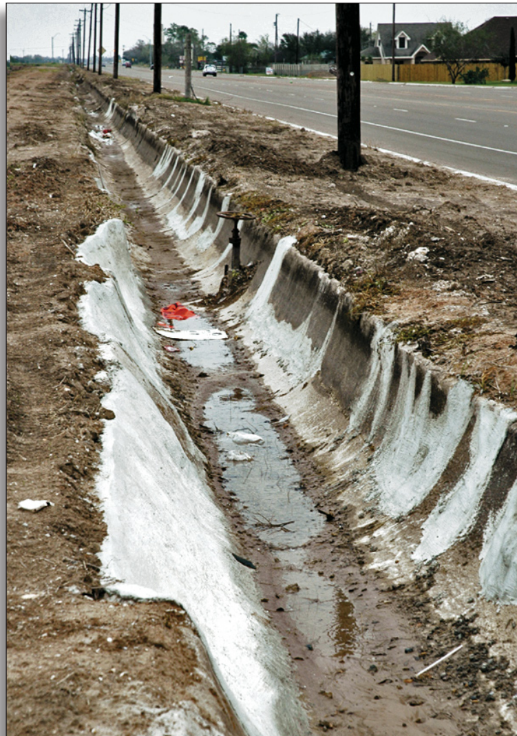
Figure 296: Modern repairs to this concrete lateral have impacted integrity of workmanship, Hidalgo County Irrigation District No. 1.
