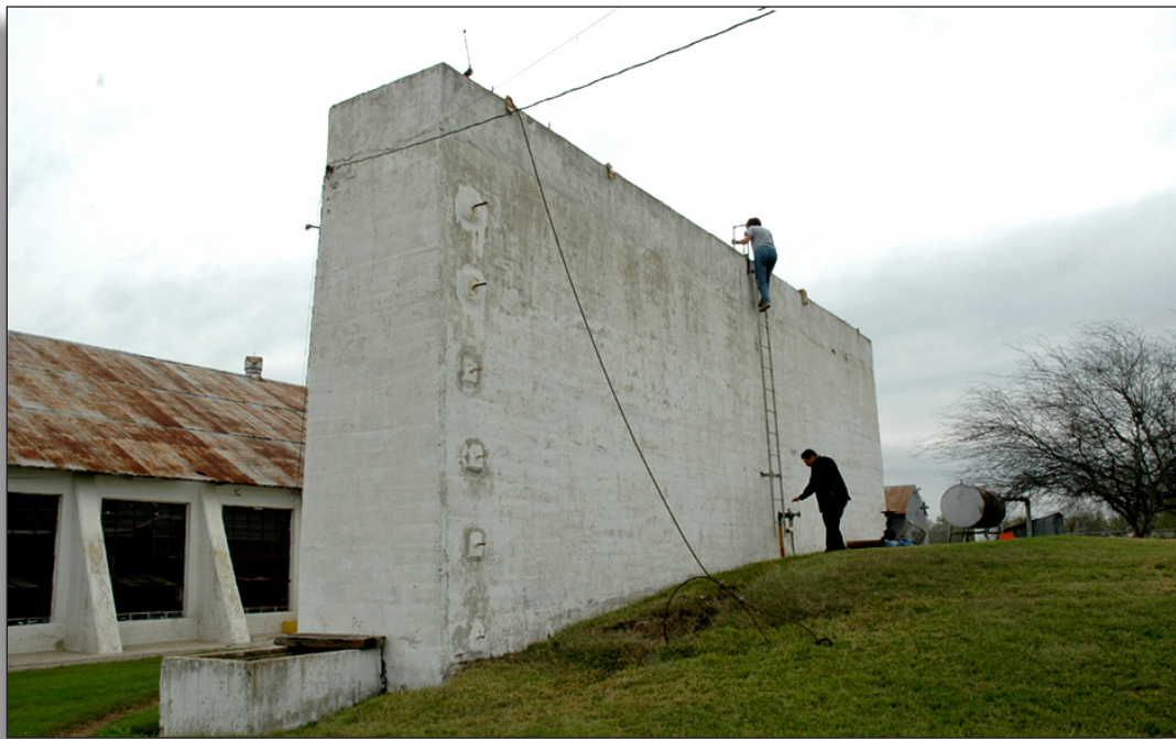
Figure 95: Surge wall (1927) at first lift pumping plant, Hidalgo County Irrigation District No. 1.
