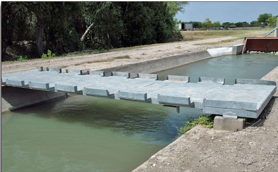
Figure 209: Foot bridge (c.2000) across Bryan Canal, Mile 2 North Road across from district office, United Irrigation District.
