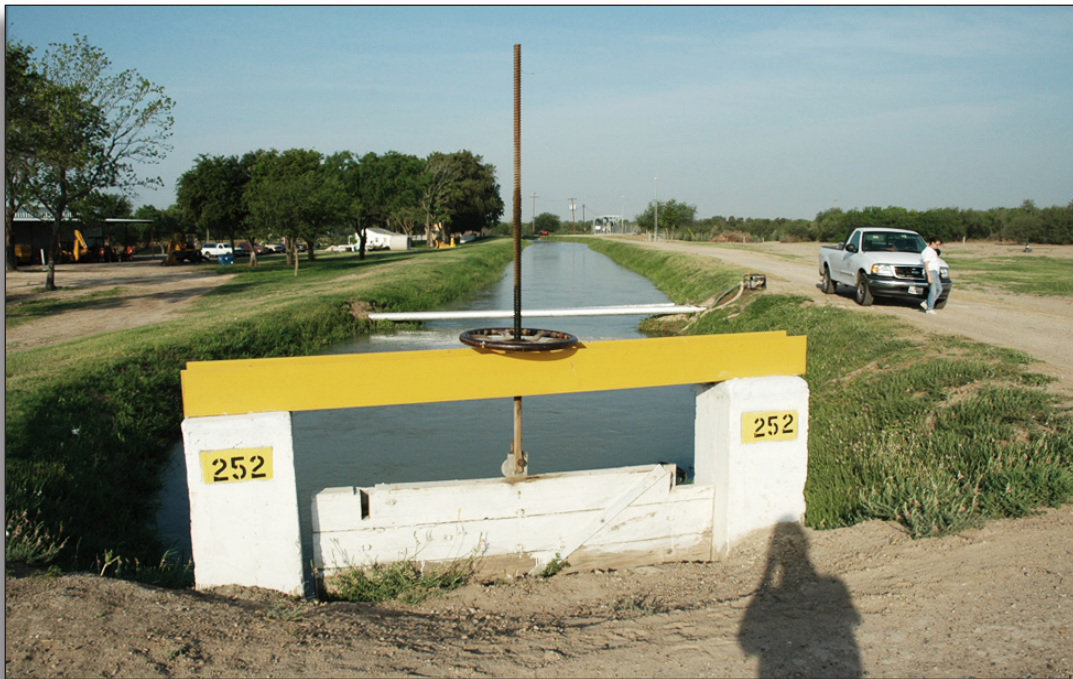
Figure 302: Workmanship is impacted by replacement of the original railroad tie crossbar with a modern steel I-beam on Check Gate No.1, Hidalgo County Irrigation District No. 3.
