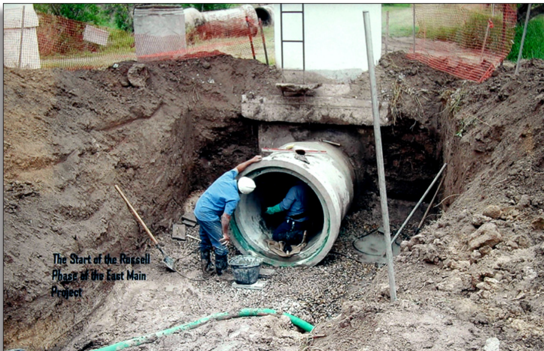
Figure 322: Installation of 48" concrete pipe with rubber gasketed joints, East Main Project (2005). Photo collection, Hidalgo County Irrigation District No. 1
