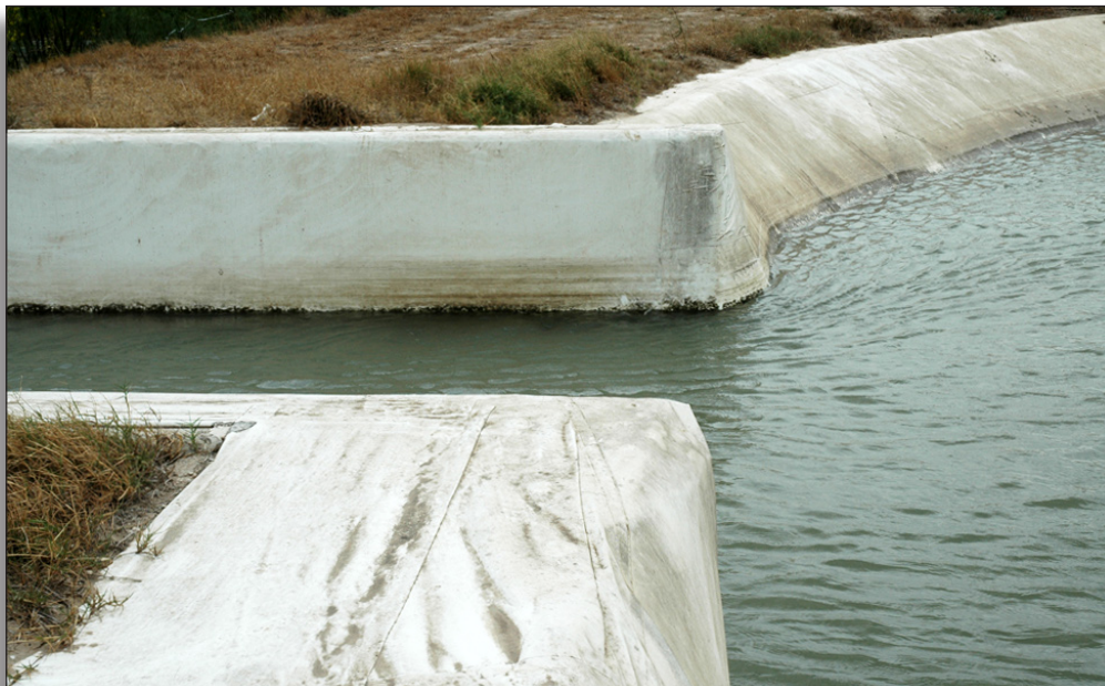
Figure 300: The use of geomembrane materials along this canal contributes to a loss of integrity of workmanship, United Irrigation District.
