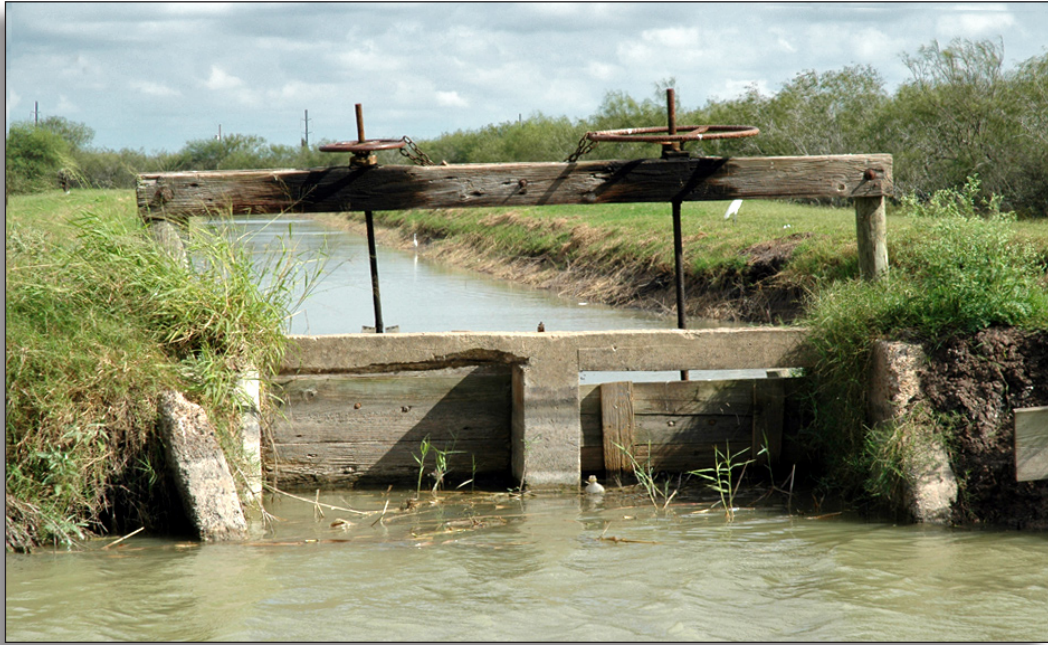
Figure 292: This wooden head gate to a lateral off main canal retains integrity of materials, Cameron County Irrigation District No. 6.
