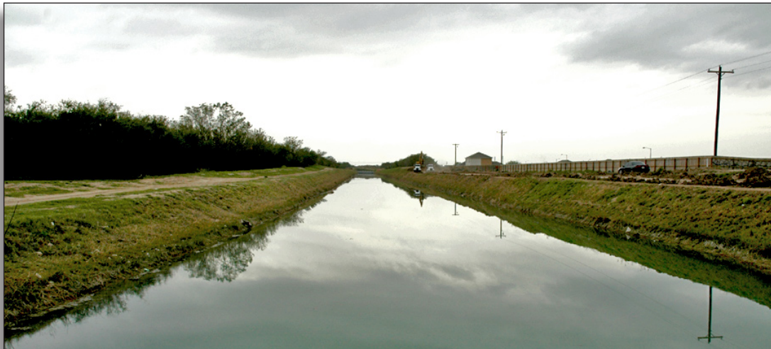
Figure 115: Edinburg Main Canal (1926) at first check gate, Los Ebanos Road, Hidalgo County Irrigation District No. 1.
