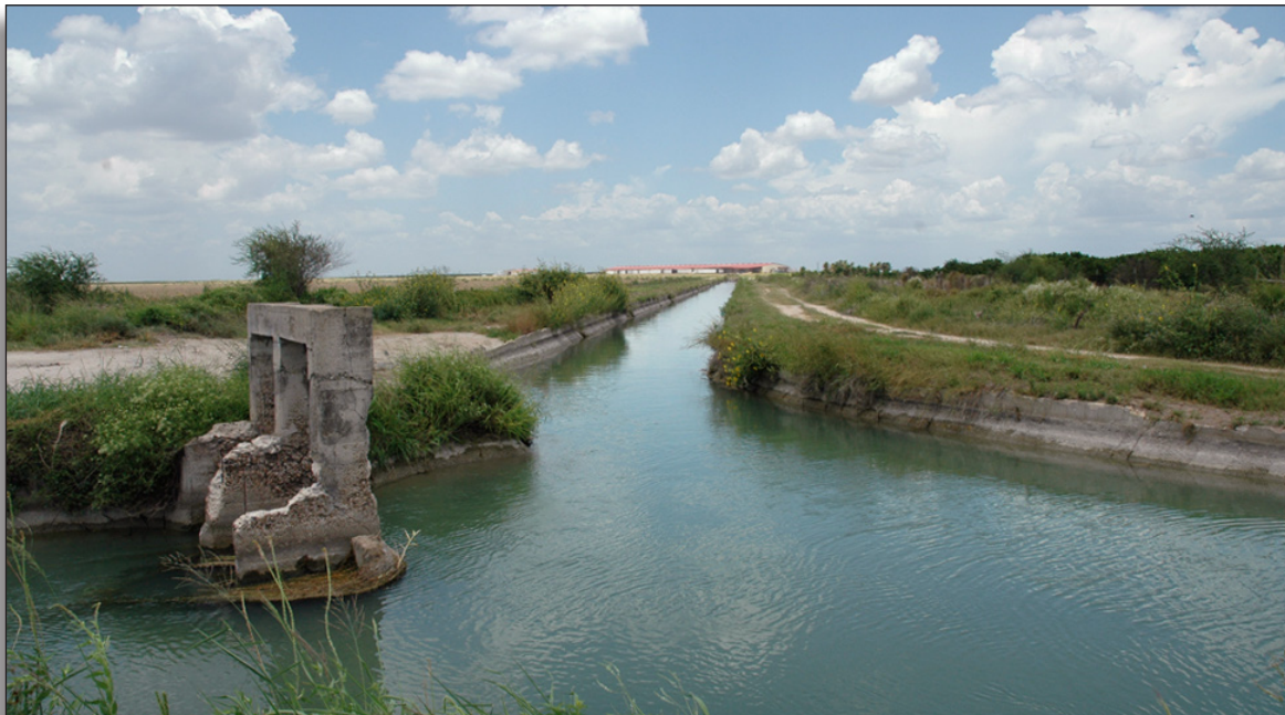
Figure 146: Old check gate north of Pump Station 13, Hidalgo County Irrigation District No. 15.
