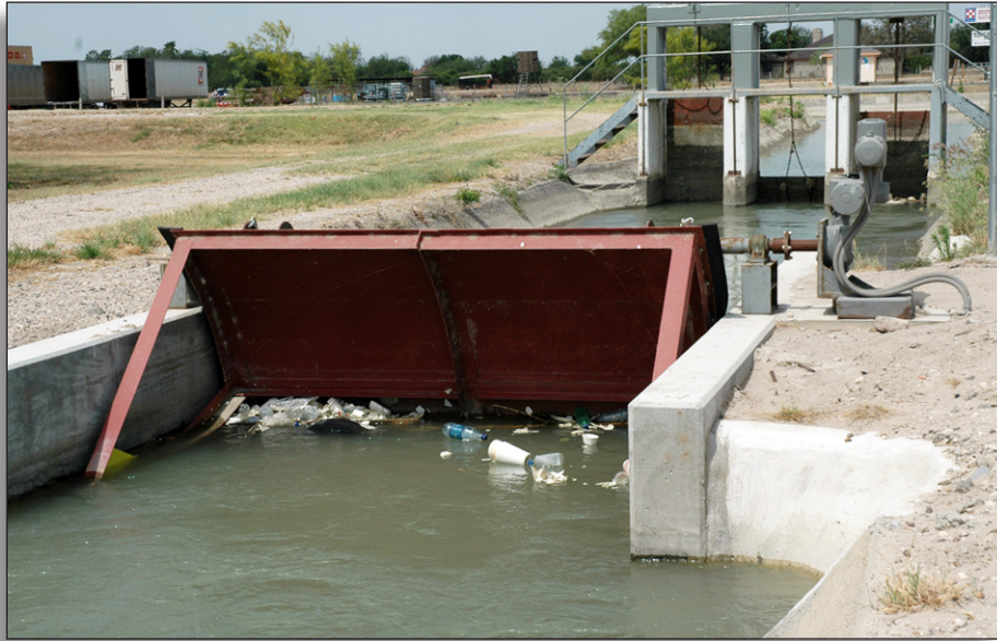
Figure 147: Electronic radial check gate (2007), United Irrigation District.
