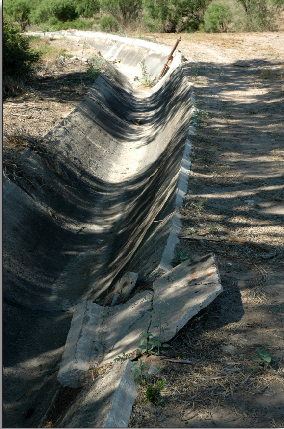
Figure 187: Abandoned sub-lateral north of Mile 6 North Road at Trosper, United Irrigation District.
