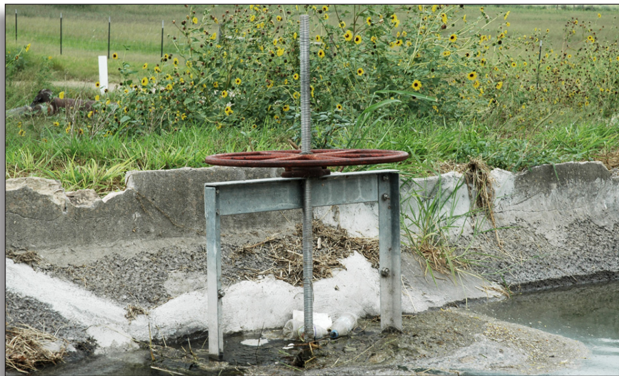
Figure 201: Turn-out gate on R-8 Canal along Mile 13 Road, Santa Cruz Irrigation District No. 15.
