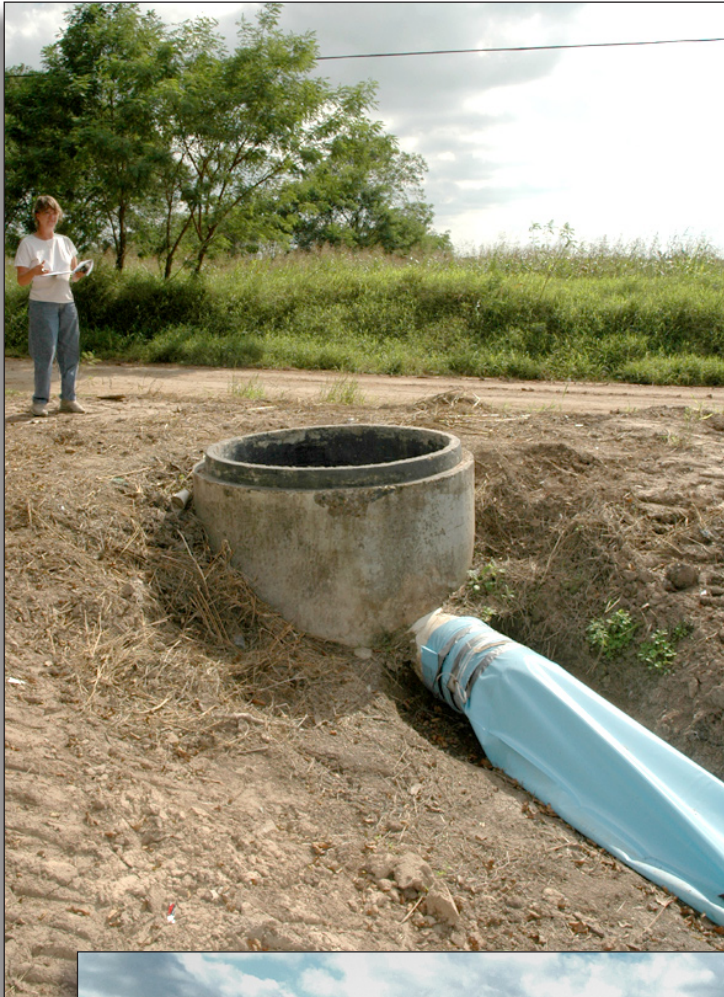
Figure 196: Poly pipe, Cameron County Irrigation District No. 6.
