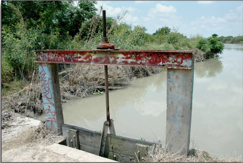
Figure 150: Head gate to lateral, Cameron County Irrigation District No. 2.
