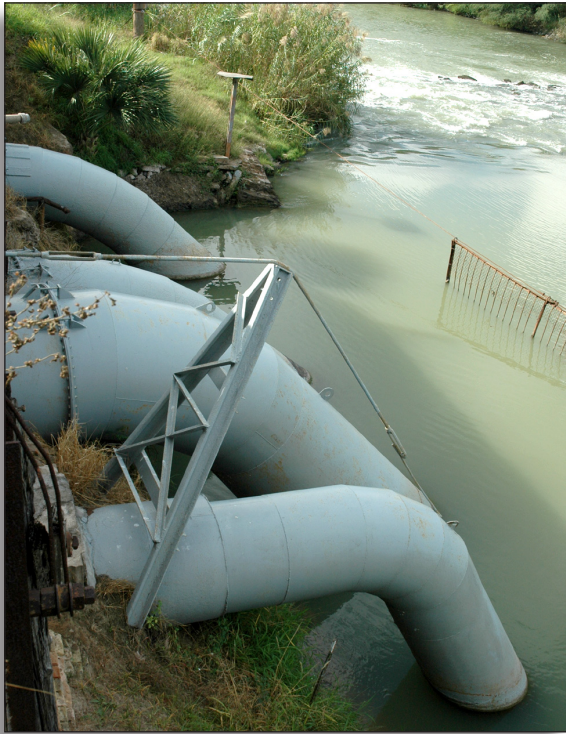
Figure 73: Inlet pipes to pumphouse, Cameron County Irrigation District No. 6.
