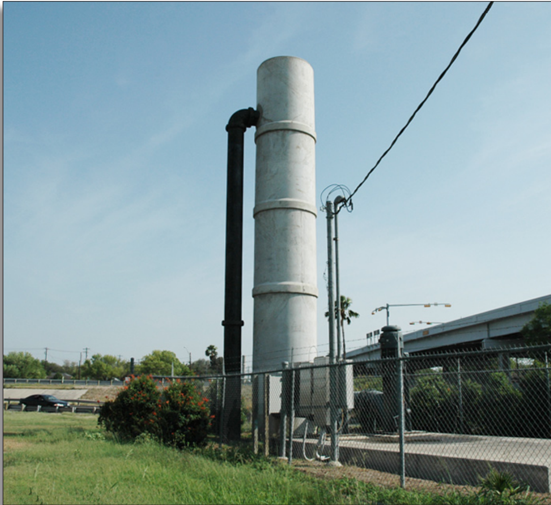
Figure 319: This second lift pumping plant lacks integrity of association because it is of modern design, it delivers water for municipal purposes and it lacks an agricultural setting, Hidalgo County Irrigation District No. 3.
