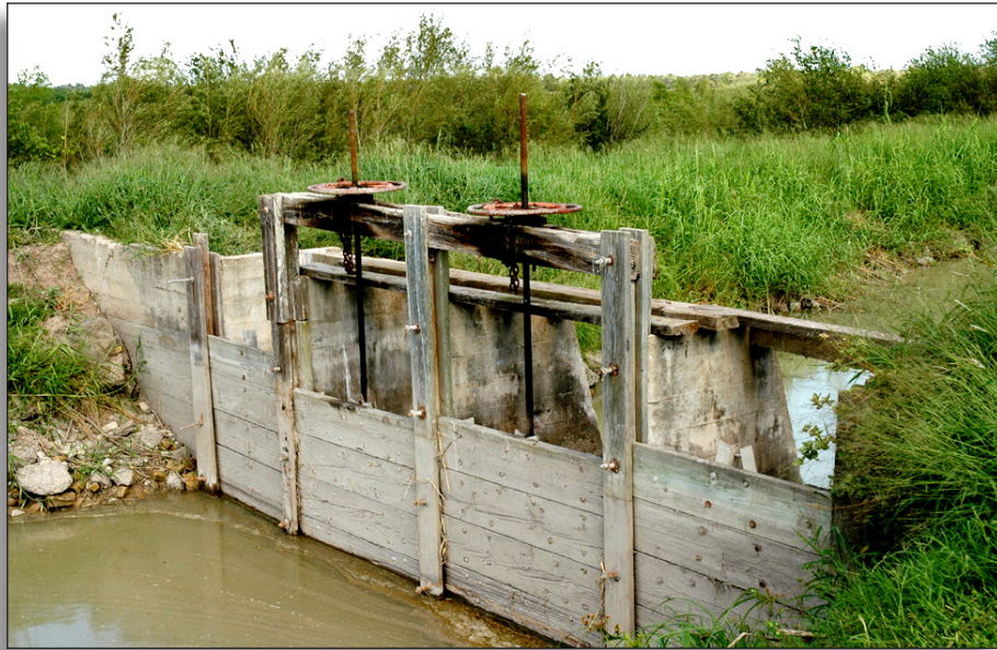
Figure 284: This check gate retains a high level of integrity and contributes to the overall integrity of design in Cameron County Irrigation No. 6.
