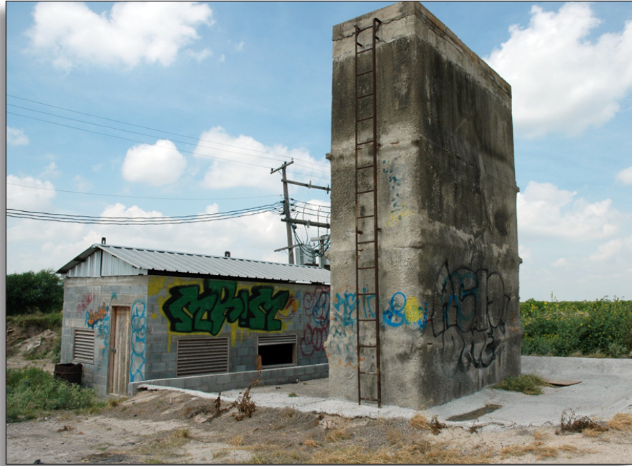
Figure 310: Unit No. 2 and the surge wall at Pump No. 8 retain setting, but have lost integrity of feeling due to years of repeated graffiti, Santa Cruz Irrigation District No. 15.
