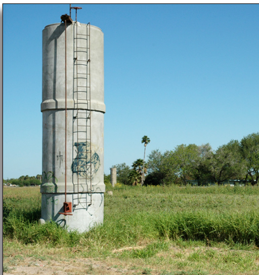
Figure 171: Gasket joint standpipe (1989) off Mile 2 North Road, United Irrigation District.
