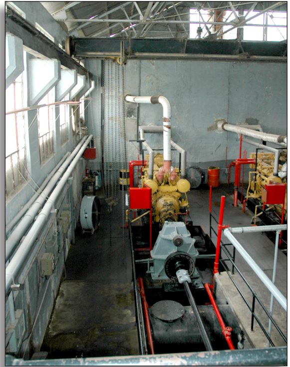
Figure 74: View of engines, first lift pumphouse, Hidalgo County Irrigation District No. 1.
