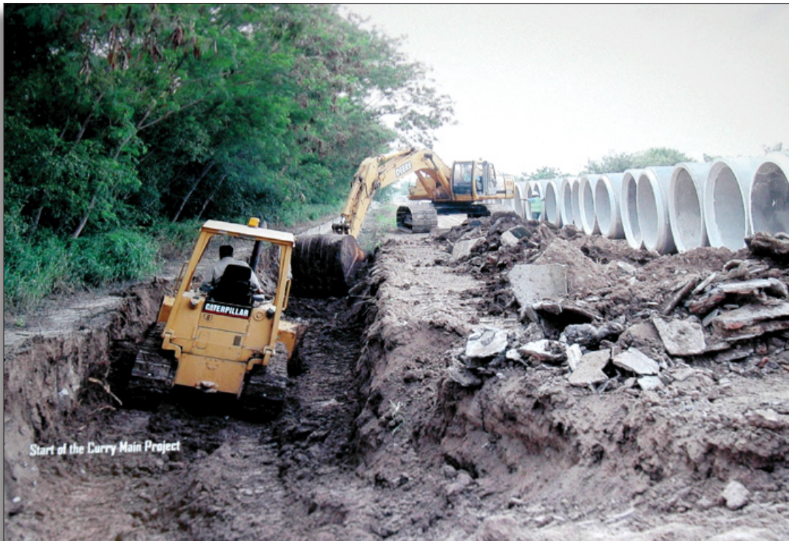
Figure 323: Initial construction on the placement of Curry Main Canal into underground pipeline (2004). Photo collection, Hidalgo County Irrigation District No. 1
