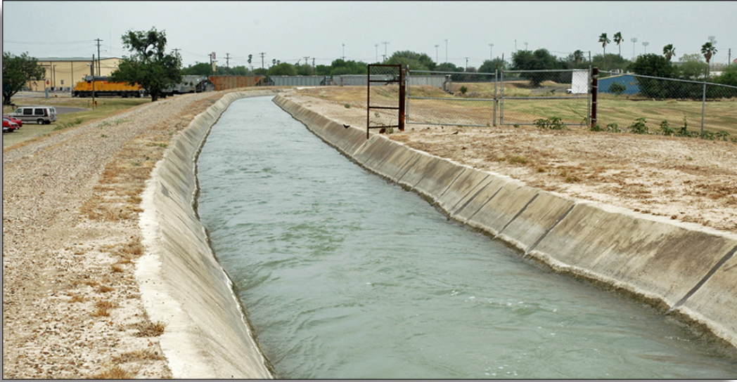
Figure 104: Concrete lined main canal (c.1930) at second lift pumping plant, United Irrigation District.
