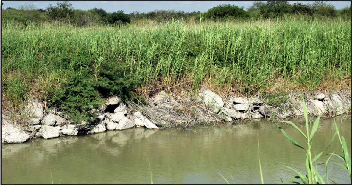
Figure 297: The lining of this earthen main canal with concrete rip-rap is a minor alteration to the integrity of workmanship, Cameron County Irrigation District No. 6.
