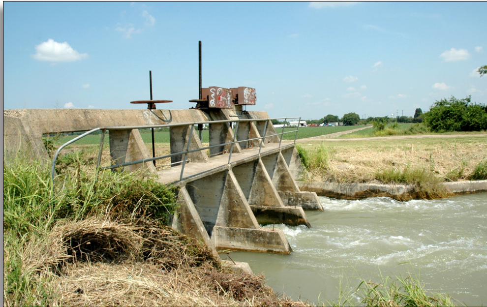
Figure 143: Motorized check gate, Cameron County Irrigation District No. 2.
