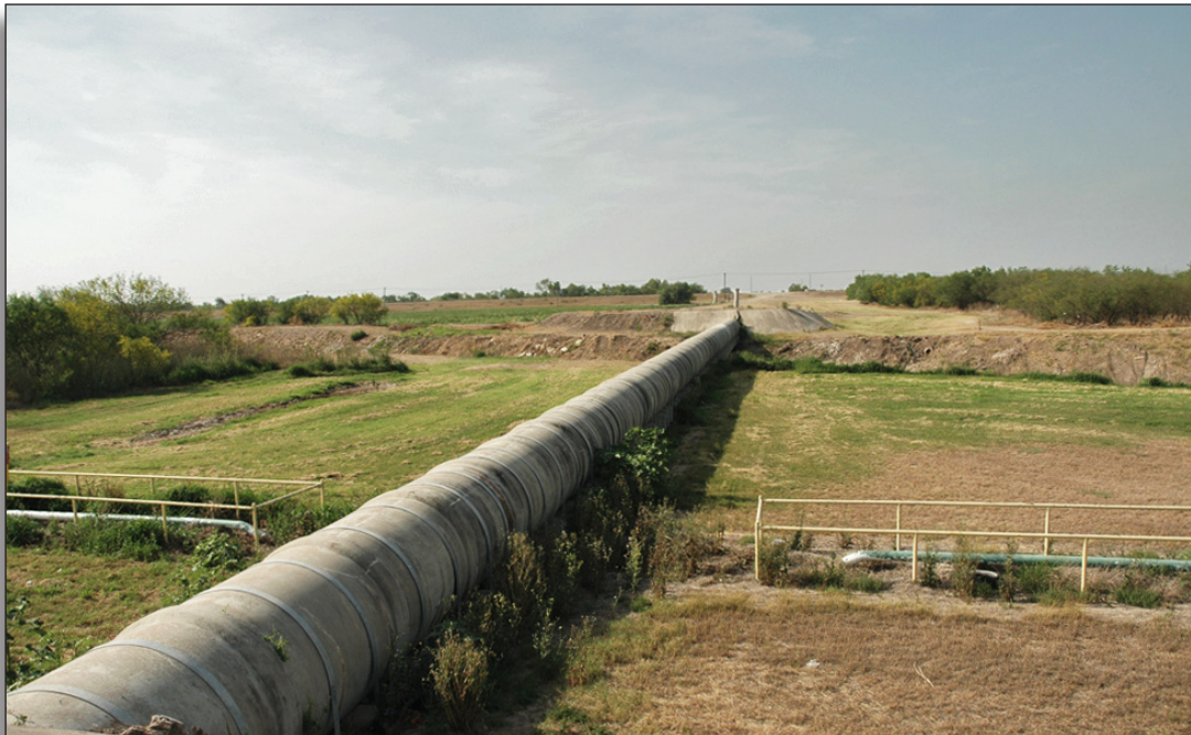
Figure 286: The design of the main canal has been altered by replacement of canal with underground pipeline and installation of a 72" pipe flume (1984) that crosses the main floodway channel, Hidalgo County Irrigation District No. 3.
