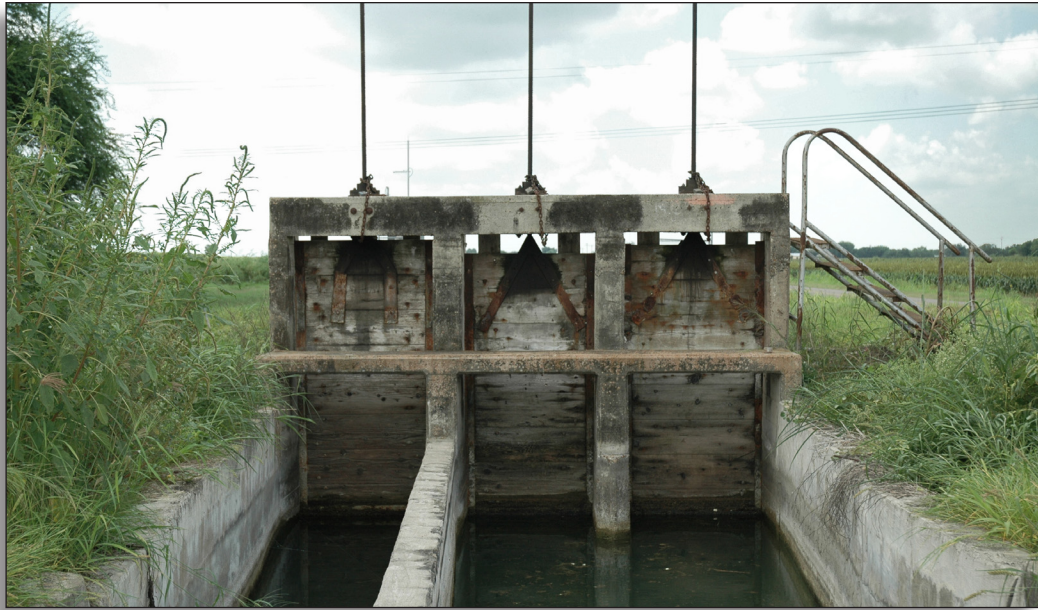
Figure 301: This head gate retains a high level of integrity of workmanship, Hidalgo County Irrigation District No. 1.
