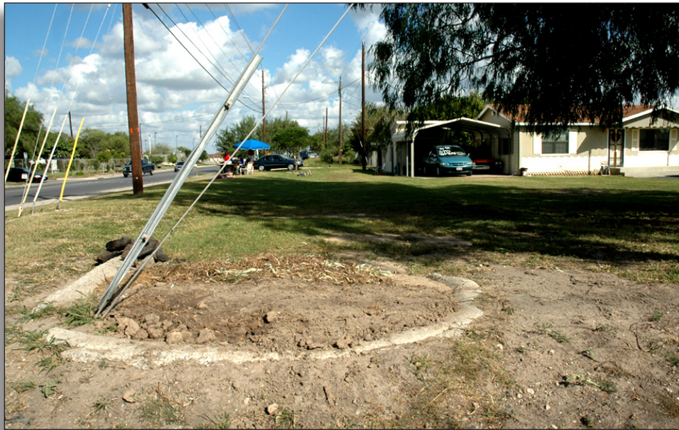
Figure 311: This abandoned canal in residential neighborhood is now filled in, resulting in loss of integrity of feeling and association, Cameron County Irrigation District No. 6.
