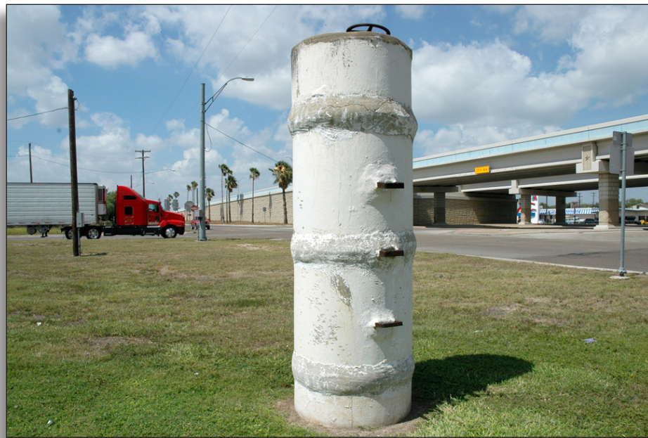
Figure 295: This standpipe retains its integrity of materials, although it has lost its integrity of setting and association, Santa Cruz Irrigation District No. 15.
