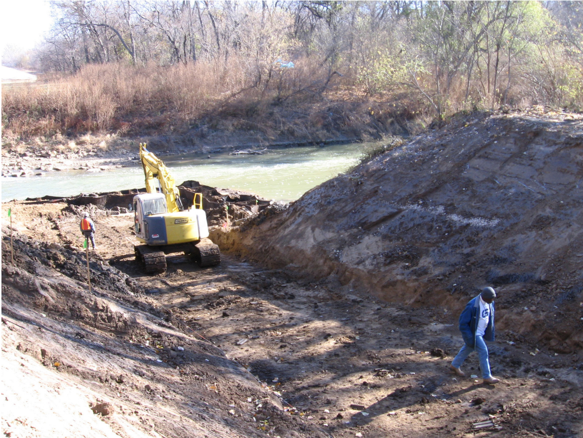
Figure 14. The boat ramp and side slopes are shown in this picture as is the initial construction of the coffer dam. The white layer in the right cut is road rock that is in the mixed overburden attributed to bridge construction and which extends to the depth that corresponds to the top of the trackhoe motor.
