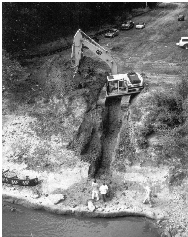
Figure 4. Trackhoe excavating Trench 2. View is to the west. Crew members are standing on the bench at the base of the slope. Trench 1 had been backfilled.
