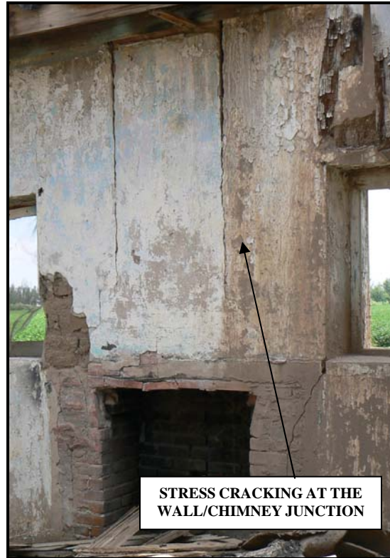
Interior view of circa 1900 dwelling in Socorro, Texas, with stress cracking/separation at the wall/chimney junction. Source: Baker, 2008.
