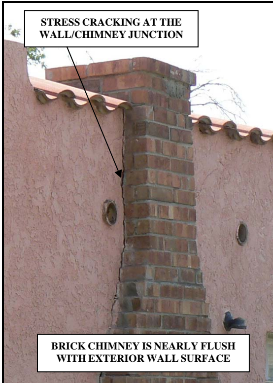
Exterior detail of circa 1940 dwelling in Ysleta, Texas. Brick chimney is nearly flush with exterior wall surface with cracking/separation at the wall/chimney junction. Source: Baker, 2008.
