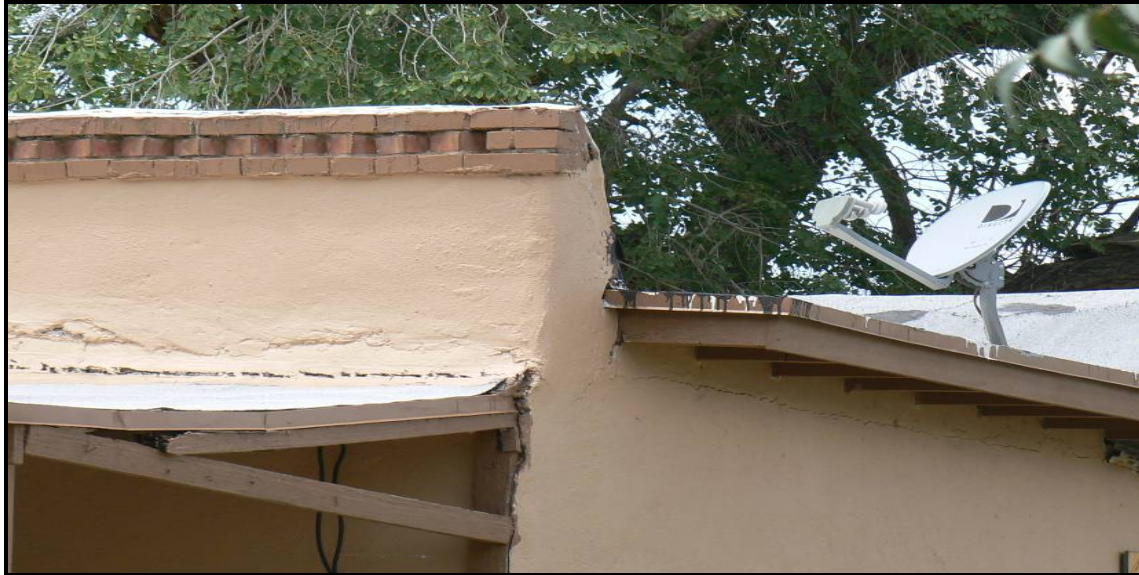
Figure 12. Detail of Territorial Style decorative brick coping, located San Elizario, Texas. Source: Baker, 2008.
