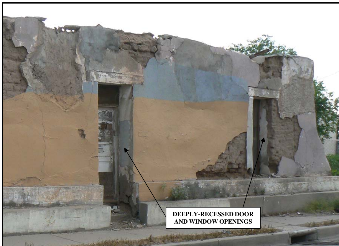
Deep window and door openings indicate that this circa 1910 building located in Socorro, Texas, is likely constructed of adobe, which is confirmed by visual inspection of the damaged walls. Source: Baker, 2008.
