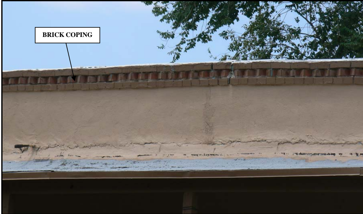
Detail of brick coping that is indicative of the Territorial Style on the parapet of a flat-roof, circa 1890, single-family dwelling in San Elizario. Source: Baker, 2008.
