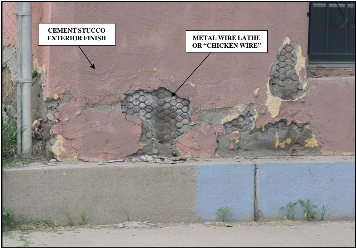
Visible wire lathe or “chicken wire” indicates cement stucco exterior wall finish, as it cement bonds poorly with adobe. Resource is a circa 1935 adobe house located in Socorro, Texas. Source: Baker, 2008.
