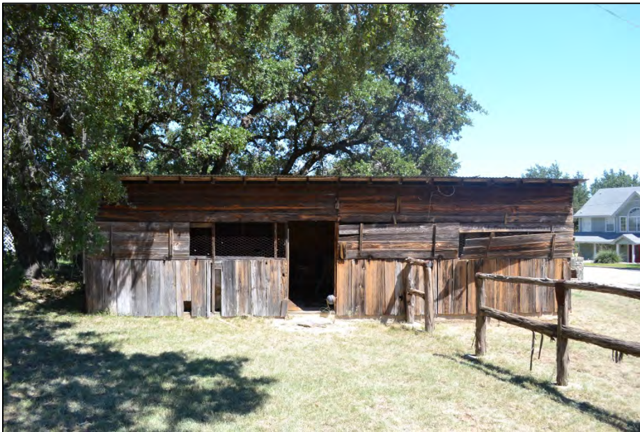
Figure 6-12. View of main façade of a chicken coop in Comal County. This image illustrates the recycling and reuse of materials that is commonly found at agricultural properties. (Source: Comal County Historical Commission.)
