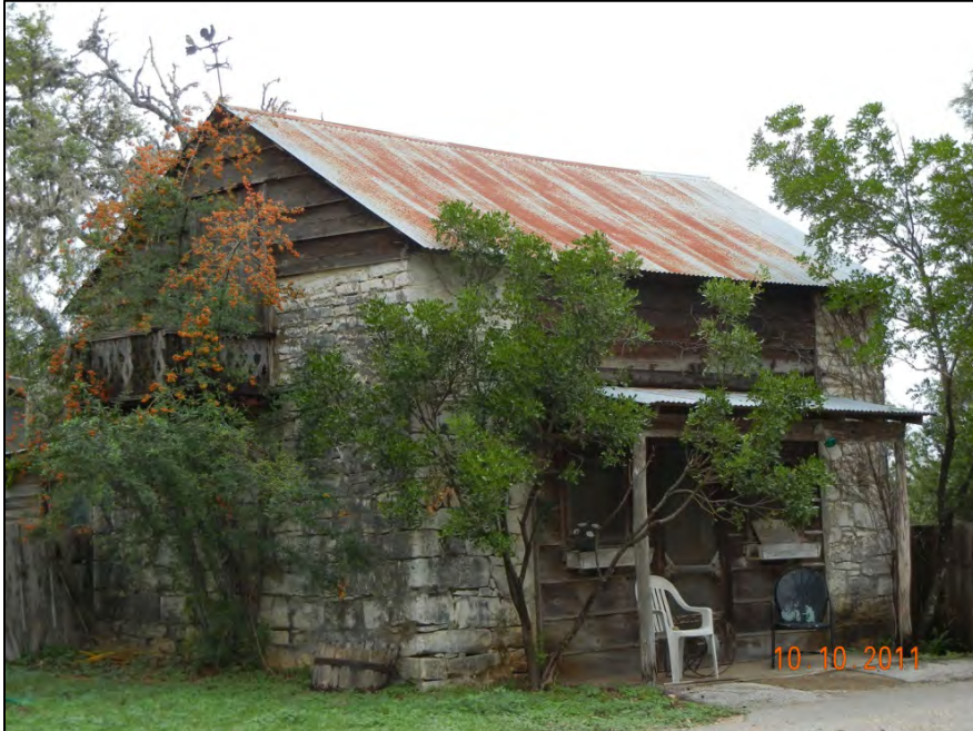
Figure 6-4. An oblique view of a stone building on the George Wilkins Kendall Homestead in Comal County. Upon his death in 1867, he was known as the “father of the sheep business in Texas.” (Source: Comal County Historical Commission.)
