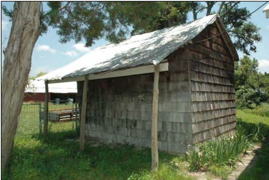
Figure 6-22. Photograph of a smokehouse associated with a nineteenth-century farmstead. Smokehouses, washhouses, spring houses, and cellars are a few examples of buildings that also reflect cultural traditions in the construction methods, forms, materials, and styles. These resources enable historians to develop a better and a more complete understanding of the history of the property and its occupants.
