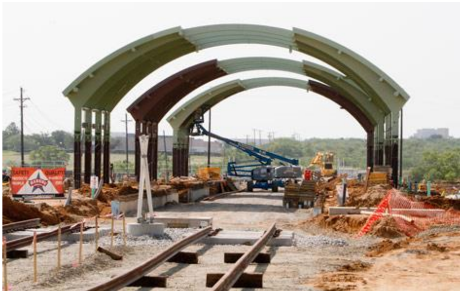
Belt Line Station is scheduled to open on December 3, 2012. The final section of the Orange Line extends from this station to Terminal A at DFW Airport
