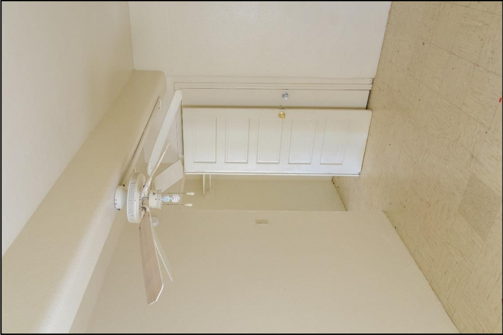
Figure B – 74: Bedroom with original six-panel door, exposed beam; Also, surface-mounted electrical conduit, view facing northwest
