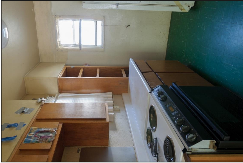
Figure B – 26: Kitchen modified to be handicap accessible; Modifications c. 1997, view facing northwest
