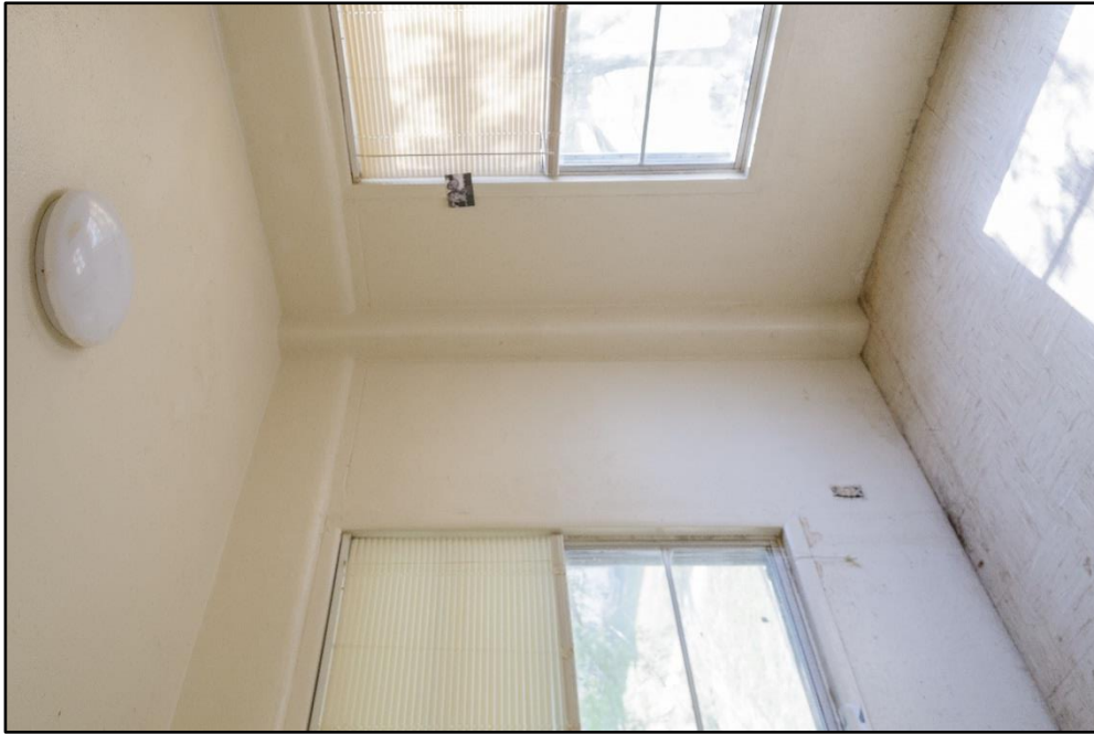
Figure B – 15: Upstairs corner bedroom with concrete beams; View facing southeast showing replacement aluminum windows
