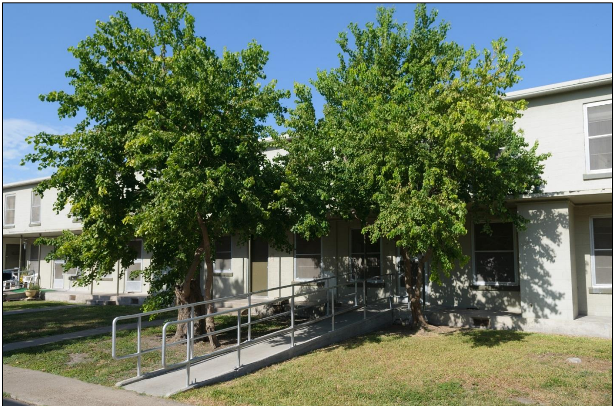
Figure 64: Ramp leading to handicap accessible unit at 1904 Fisk Ct. in Building No. 17, Type A
