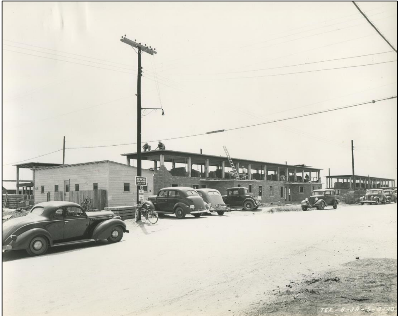
Figure 53: Installation of hollow clay tile cladding over concrete structure on Winnebago Street on May 8, 1940
