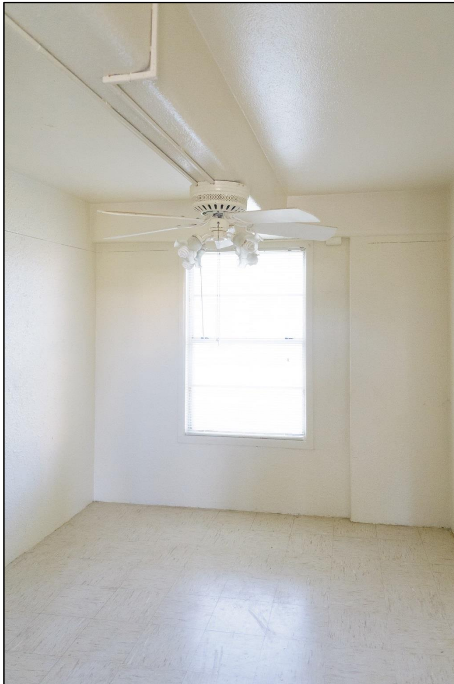
Figure B - 67: Bedroom with exposed concrete structure, surface-mounted electrical conduit; Also ceiling fan shown, view facing southeast
