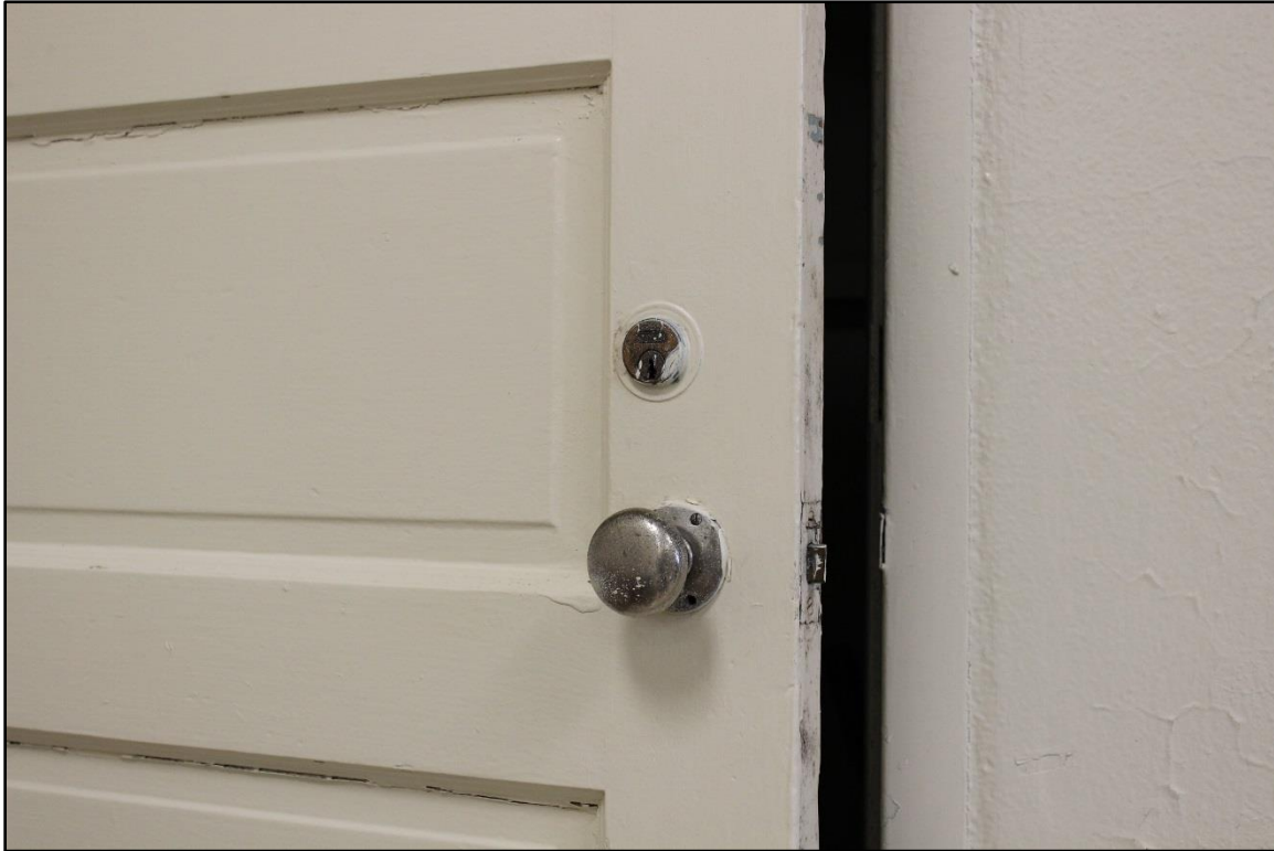
Figure 62: Example of exterior view of Yale-brand rim lock thought to be typical original lock
