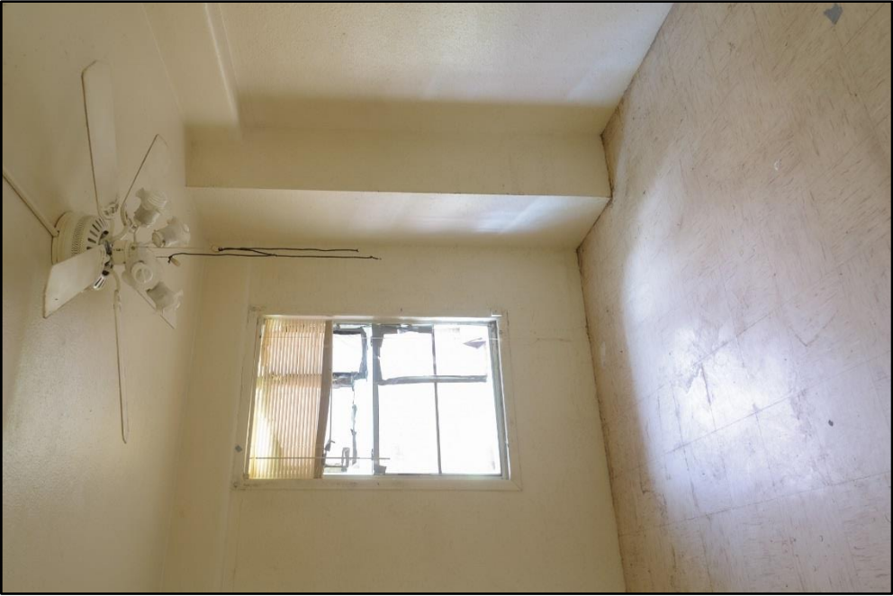
Figure B – 25: Bedroom with exposed concrete structure; Also, surface-mounted electrical conduit, view facing southwest
