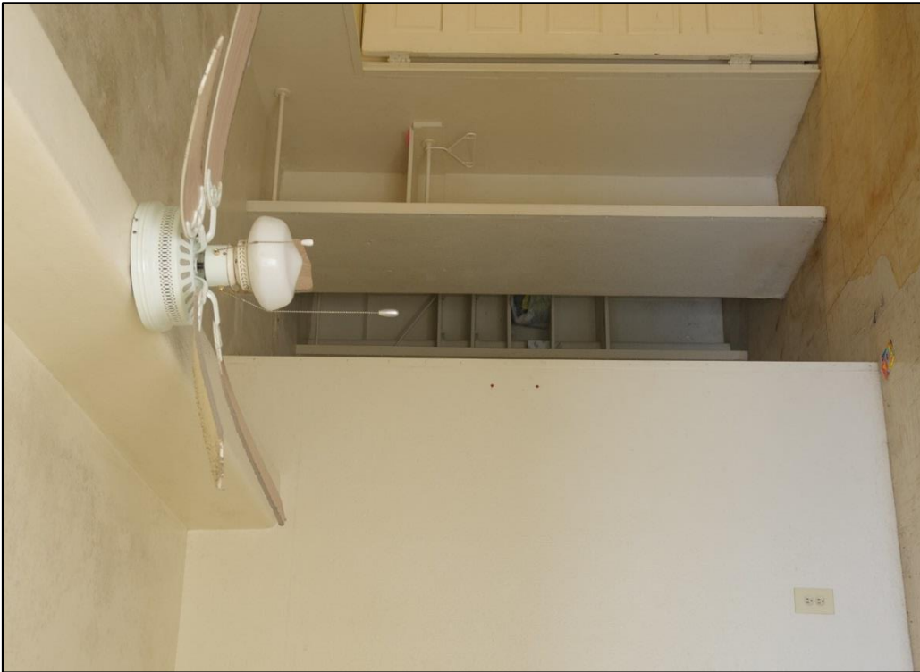
Figure 59: Living room coat closet with no door door to bedroom to the right
