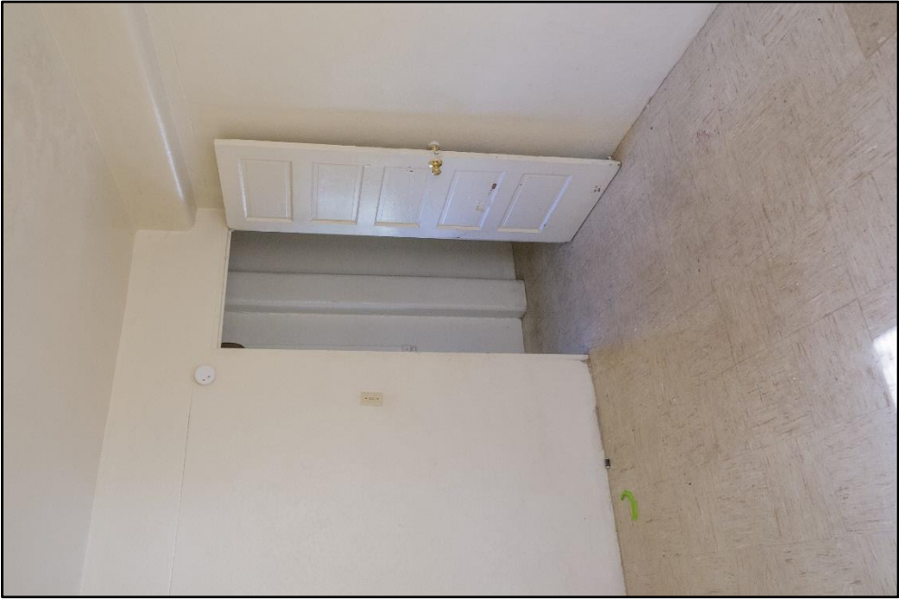
Figure B – 14: Middle bedroom with exposed concrete structural beams; Original, six-panel, bedroom door, view facing northeast
