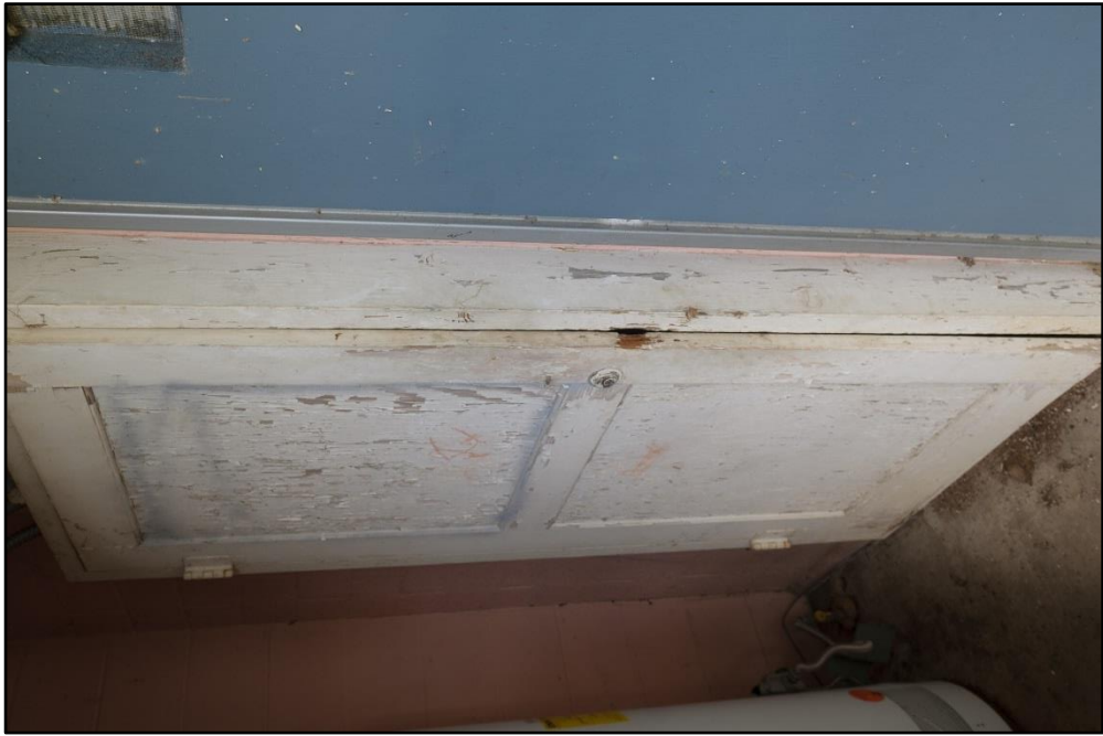
Figure B – 17: Original electric service closet on Building 14; Original two-panel wooden door, view facing northwest
