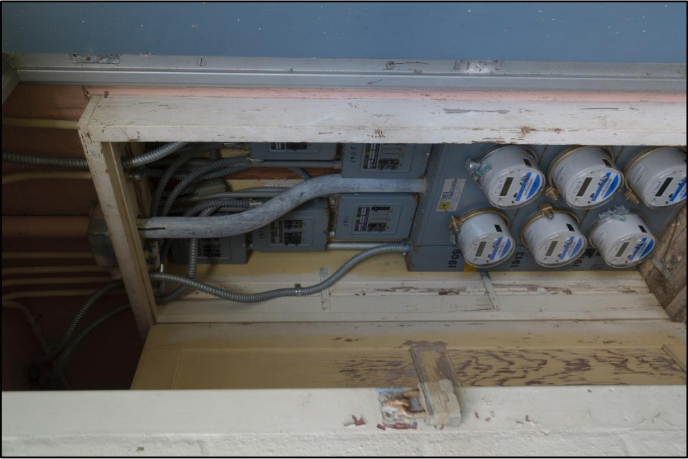
Figure B – 18: Interior of typical electrical closet, view facing northwest; Electrical closet located inside water heater closet addition
