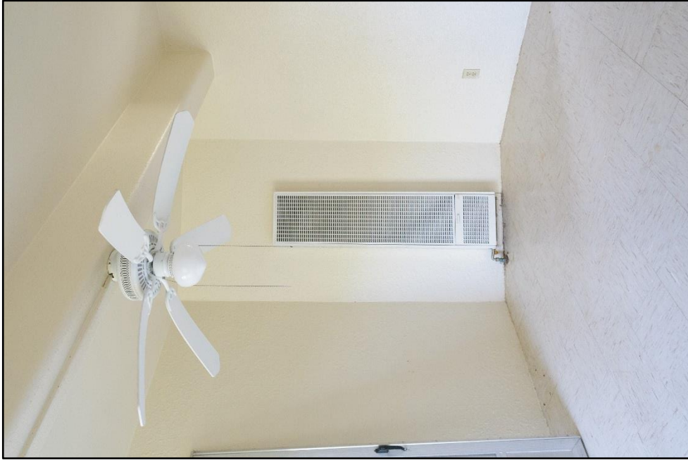
Figure B – 61: Living room with corner wall heater; Ceiling fan mounted on concrete beam, facing northwest
