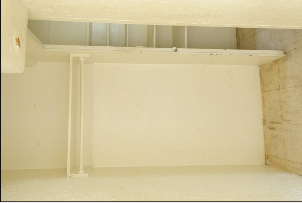
Figure B – 23: Original design hall closet without door; Linen shelves to right beyond typical plaster wall, view facing west
