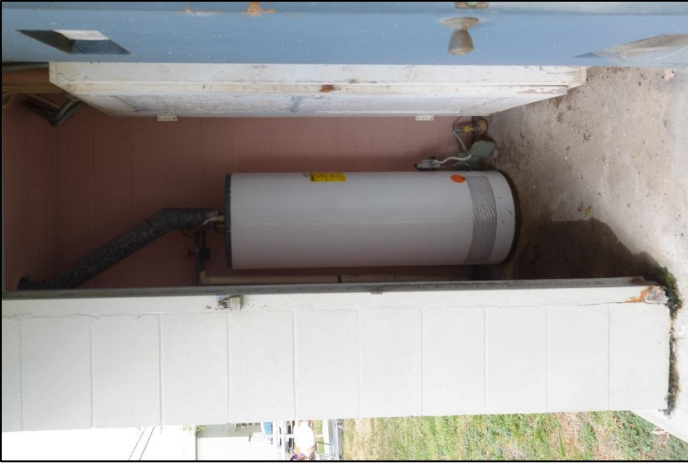
Figure B – 16: Water heater closet addition with electrical closet; Electrical closet to the right, view facing west
