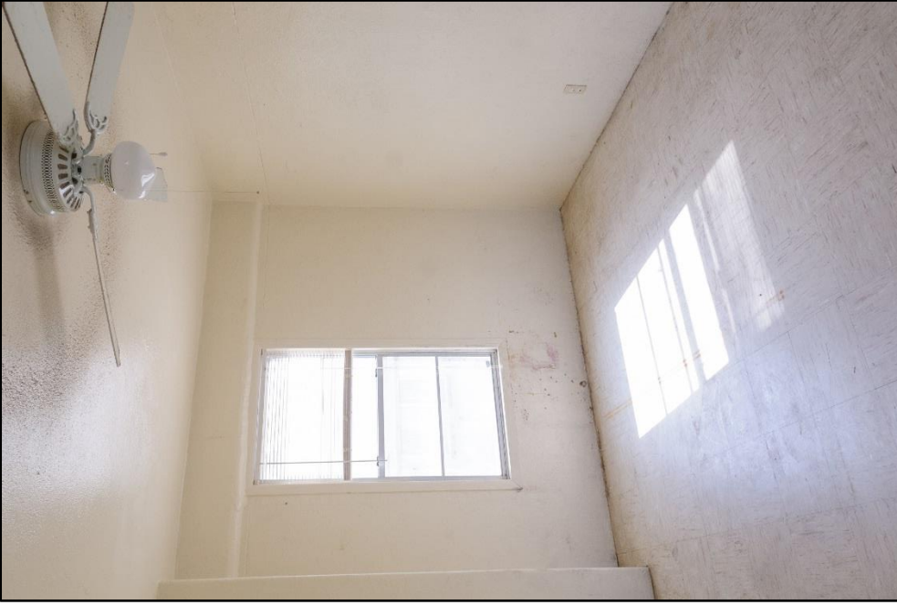
Figure B – 12: Largest bedroom with concrete structural beams visible; View facing southwest
