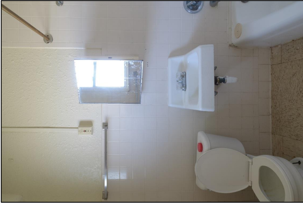
Figure B – 65: Bathroom with c. 1997 modernized fixtures and tile; View facing east Figure B – 66: Bedroom toward closet (with door added), facing northeast; Original bedroom door and hall beyond with linen shelves
