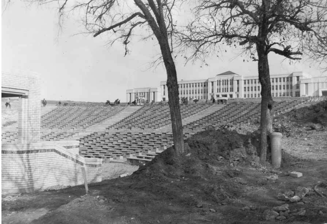
This amphitheater at North Side Senior High School was one of many projects Morrison designed and oversaw for the school district in the 1930s.
