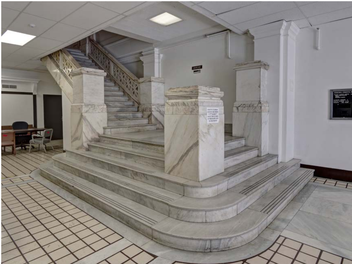
This marble stair on the fifth floor of the Criminal Courts Building was removed during the building’s renovation, but the components have been stored.
