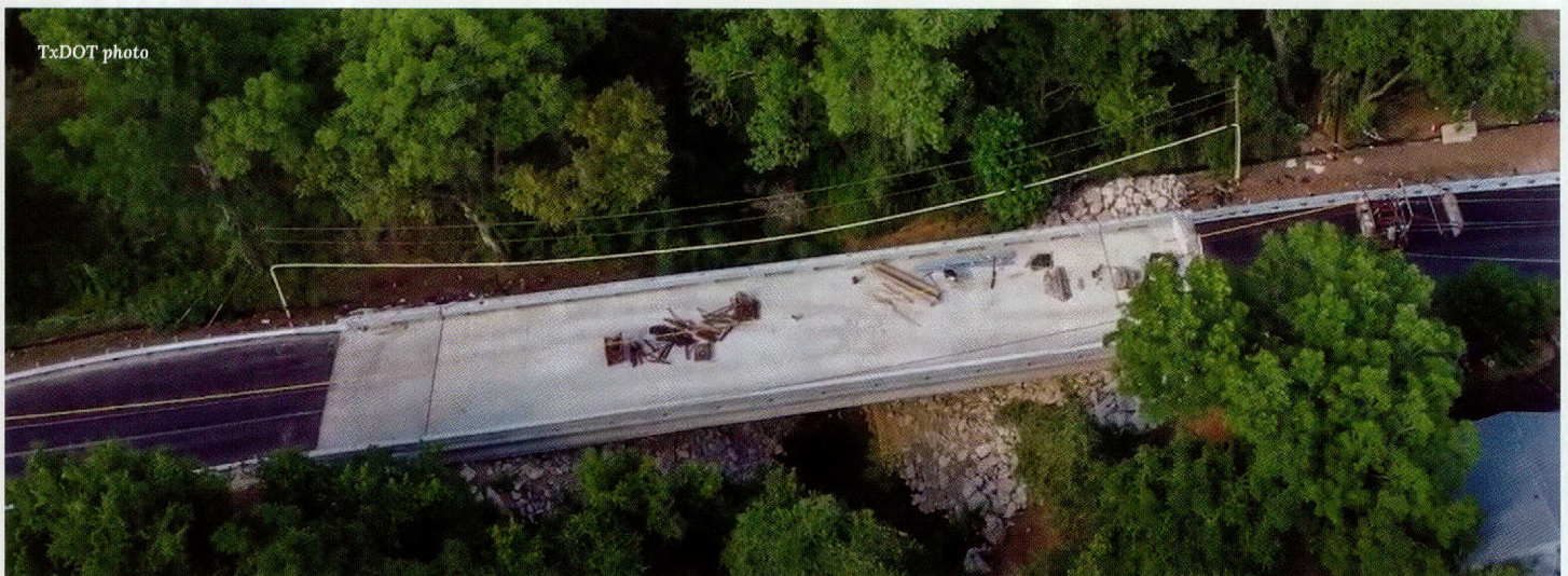
The Fourth Avenue Bridge over Gazley Creek in Smithville officially opened to traffic in August.
